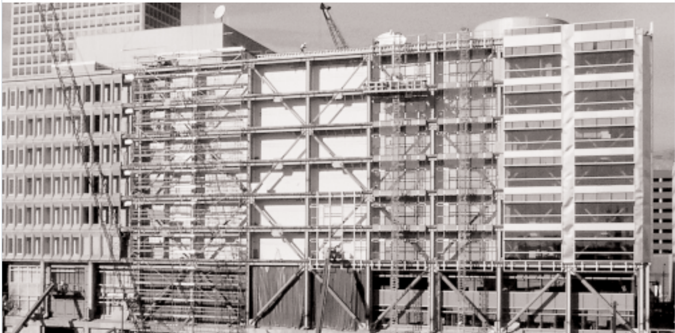
The W.F. Bennett Federal Building in Salt Lake City is the first federal building to use buckling-restrained brace technology.
