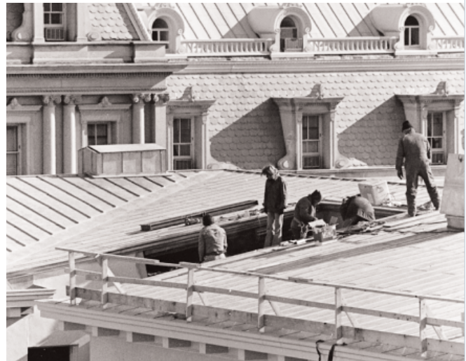
Workmen on the roof of the Winder Building, Washington, D.C. install a window as part of a renovation project.
