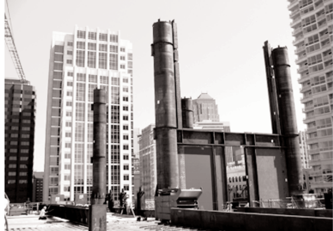
The recently completed Seattle Courthouse Steel Plate/Composite Concrete Shear Wall System during construction.
