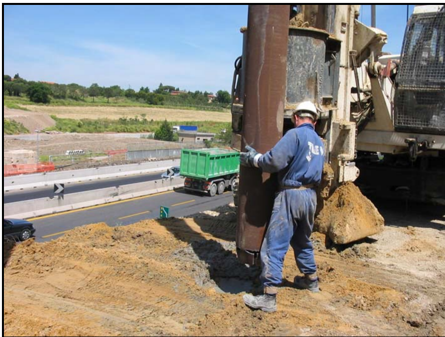
Figure 4.25: Use of Steel Pipe to Reinforce a CFA Pile for a Wall
