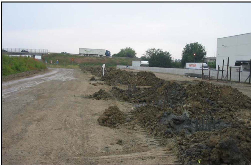
Figure 3.6: CFA Piles for Soundwall (at right) along Highway (out of view to left)
