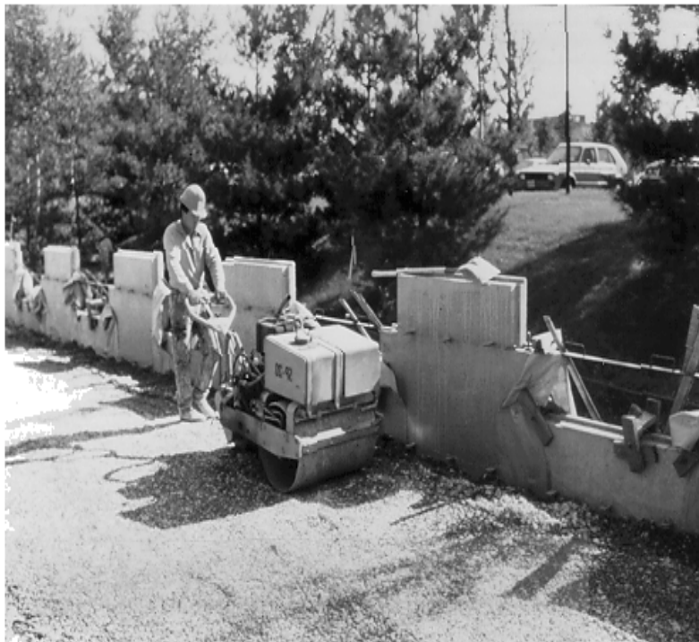
Figure 84. Compaction equipment showing: a) large equipment permitted away from face; and b) lightweight equipment within 1 m of the face.
