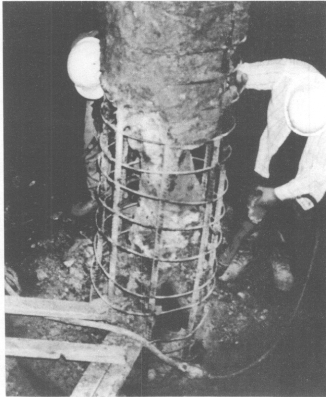
Figure 17.2. A severe defect that can likely be detected by sonic echo testing
