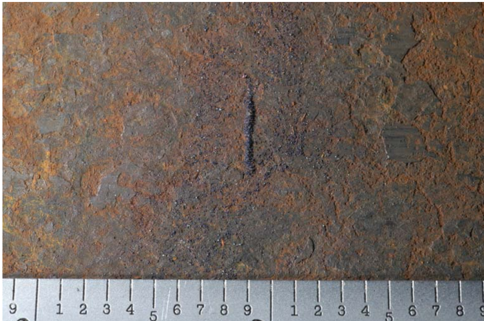
Figure 12: Shows the inside surface of the leak
