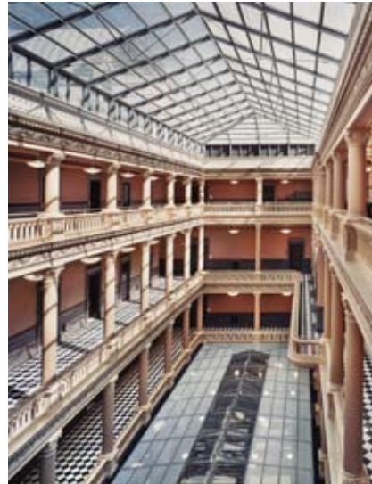
FIGURE 4 Include repair or replication of skylights concealed by previous roof repairs to improve the marketability of windowless workspaces.
