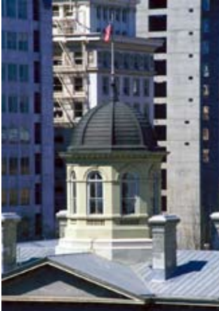
FIGURE 3 Repair and installation of slate, clay tile and metal roofing requires specialized construction skills. Competency of Restoration Specialist requirements reduce GSA risk by limiting competition to firms having successful experience with historic building projects of comparable complexity.
