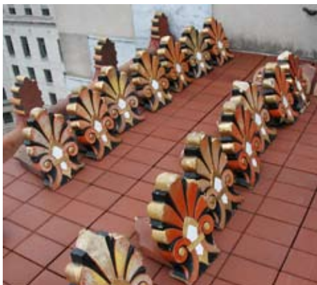
FIGURE 2 Damaged or missing features such as decorative acroteria should be repaired or replicated as part of a major roof project.
