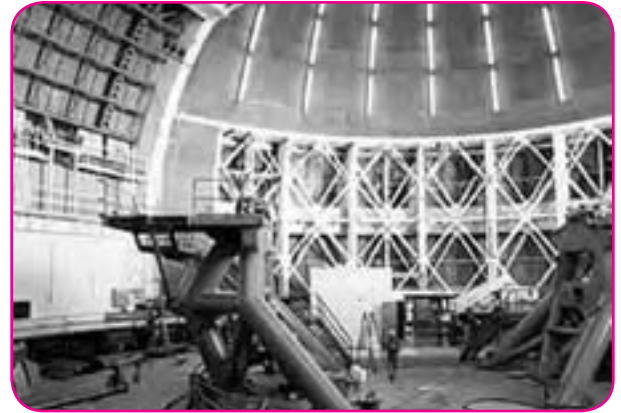
Installation of the Gemini North telescope. The Gemini facility is an international partnership for which NSF acts as the executive agency. Credit: NOAO/AURA NSF
