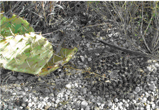
Nipple cactus and prickly pear to be saved by hand salvage prior to construction disturbance along Walnut Canyon Road. (NPS Photo by Meredith Gosejohan)
