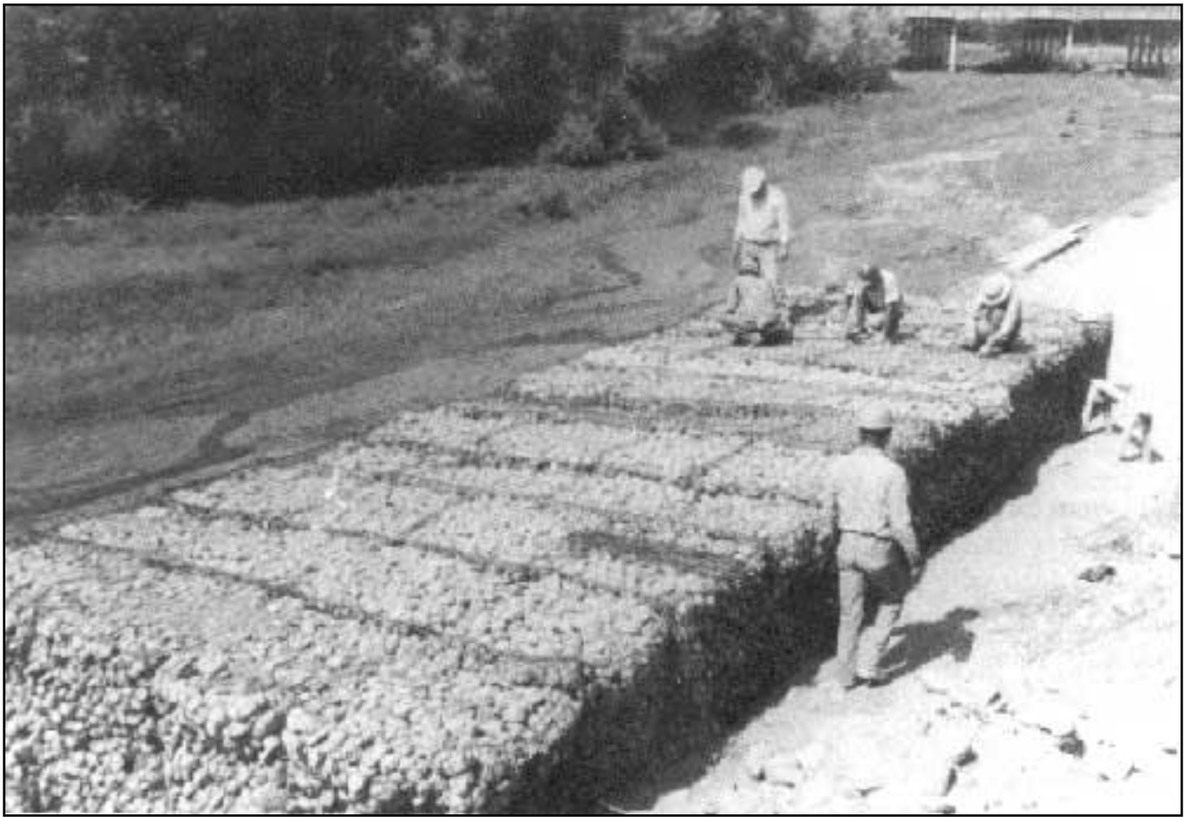
Figure 47. Creating gabions in the Pueblo Colorado Wash in an attempt to prevent erosion, 12 July, 1974. NPS photo by Mike Varela. HUTR Neg. R151#19.
