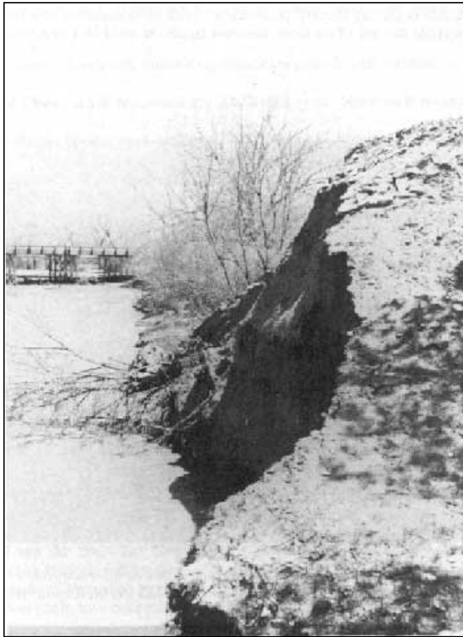
Figure 46. Erosion along the Pueblo Colorado Wash in May of 1973. This is the Wide Reed Ruin Site. NPS photo. HUTR Neg. R146#4.
