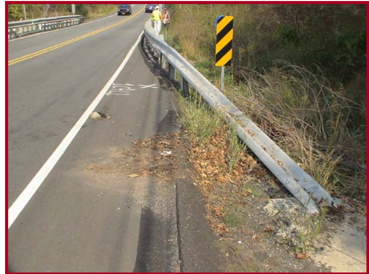
Guide rail at Deep Creek with obsolete end treatment. Hazard markers located behind guide rail
