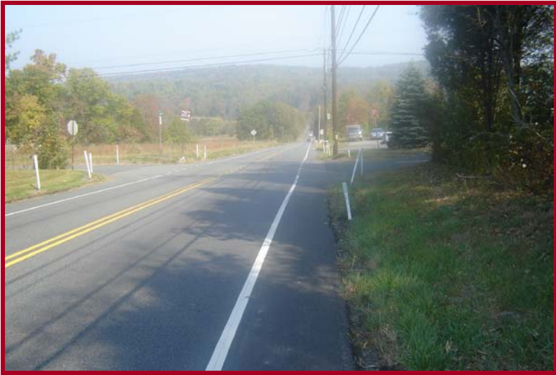
PA 663 at the Little Road intersection – pavement drop off damaged delineators
