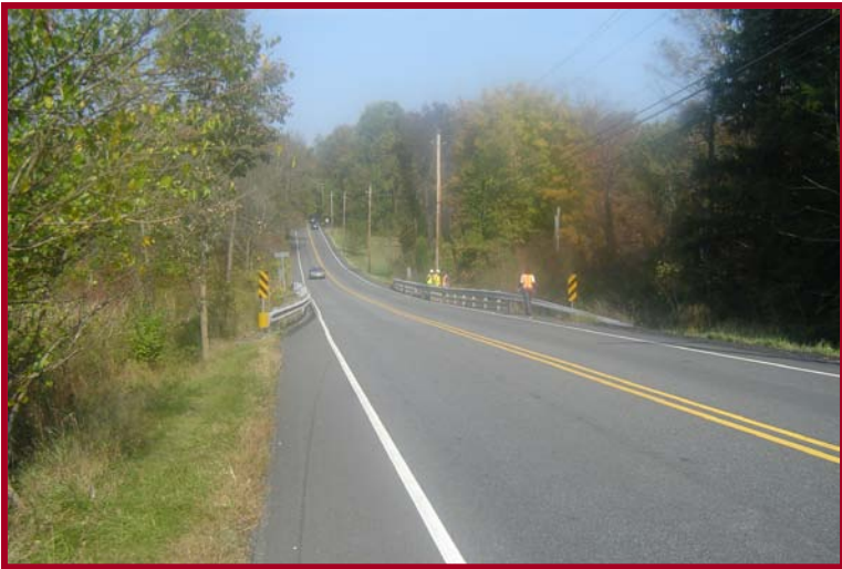
Box culvert over Deep Creek – misplaced hazard signs and obsolete guide rail end treatment on the right
