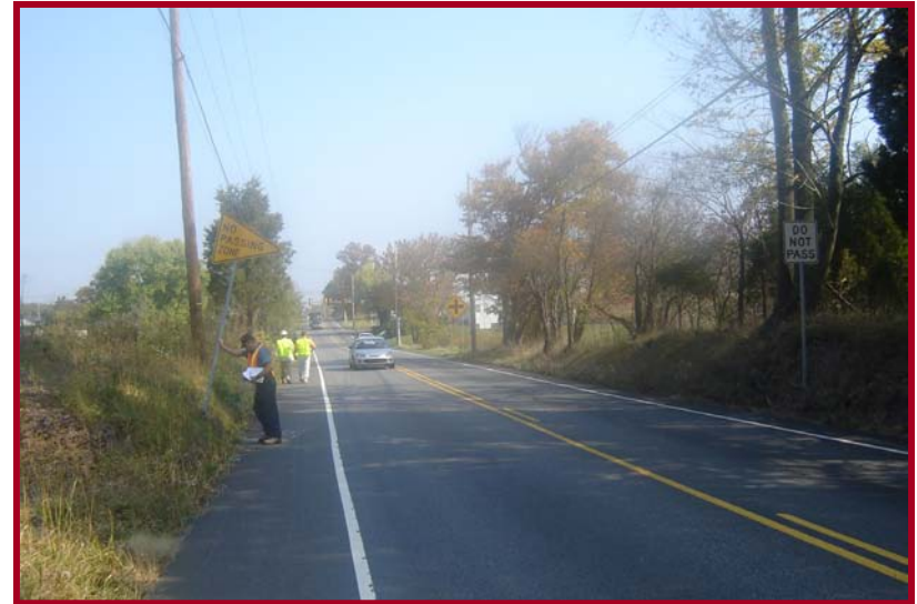
Leaning "No Passing Zone" sign approaching Hoffmansville Road intersection
