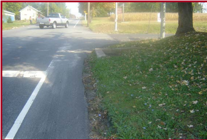
Shoulder drop-off at the southeast corner of the Hoffmansville Road intersection. Concrete headwall for drainage inlet - hazard
