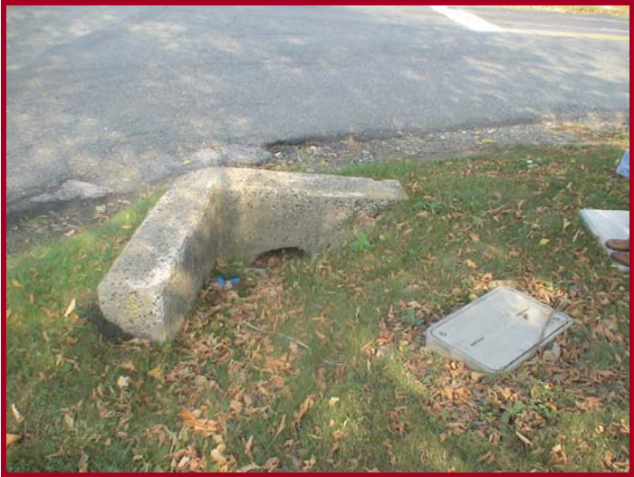
Concrete headwall for the drainage inlet at the south east corner of the Hill Road intersection
