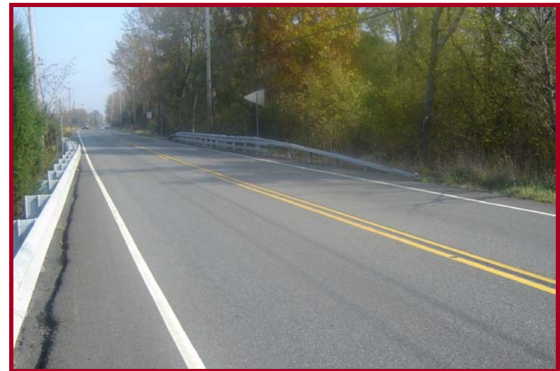
Narrow bridge on PA 663 between Hoffmansville Road and PA 73. Passing zone extends on to the bridge.
