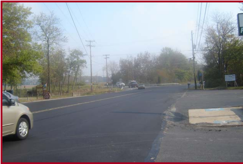
Restaurant/camp ground driveway on PA 73 (Big Road) just west of Layfield Road (PA 663) is not defined.
