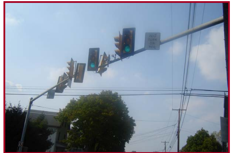
Signal heads and mast arms at PA 663/Kutztown Road intersection
