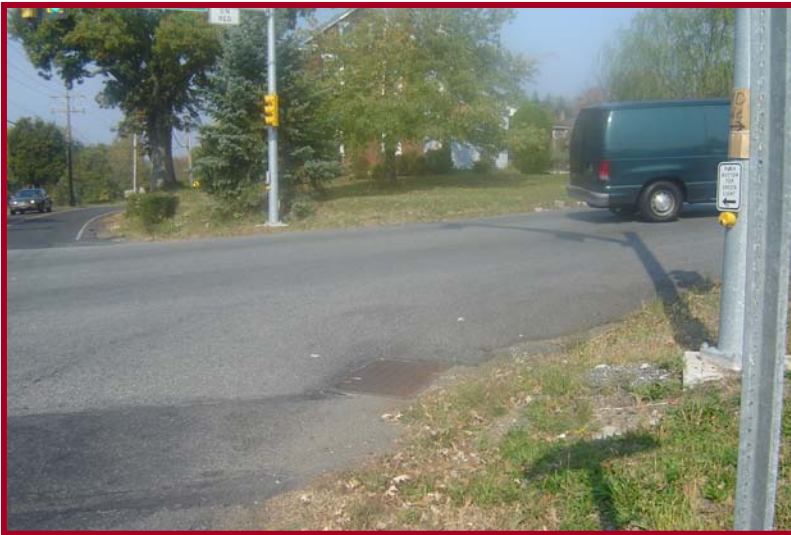
Drainage inlet on the northeast corner of the Hoffmansville Road intersection
