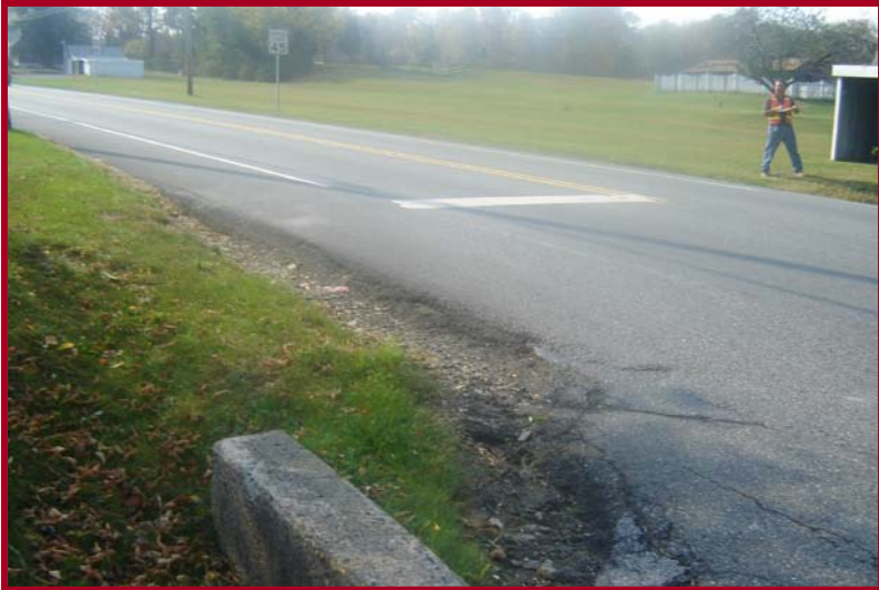
Pavement drop off at the south east corner of the Hill Road intersection
