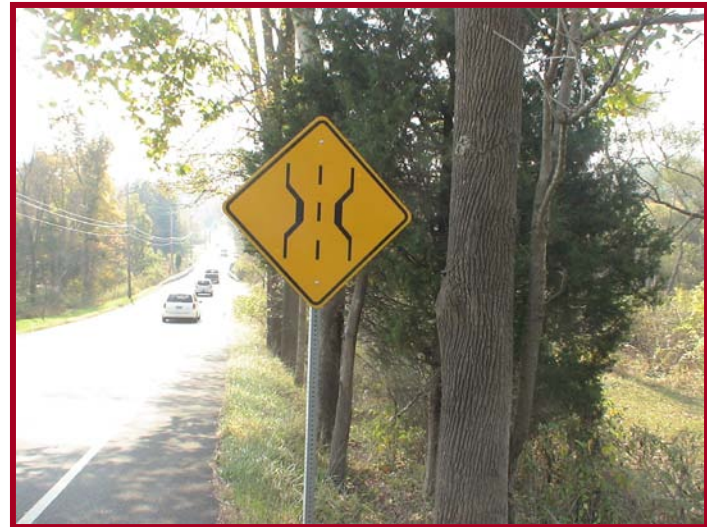
Advance warning “bridge” sign for box culvert over Deep Creek – too close to the culvert
