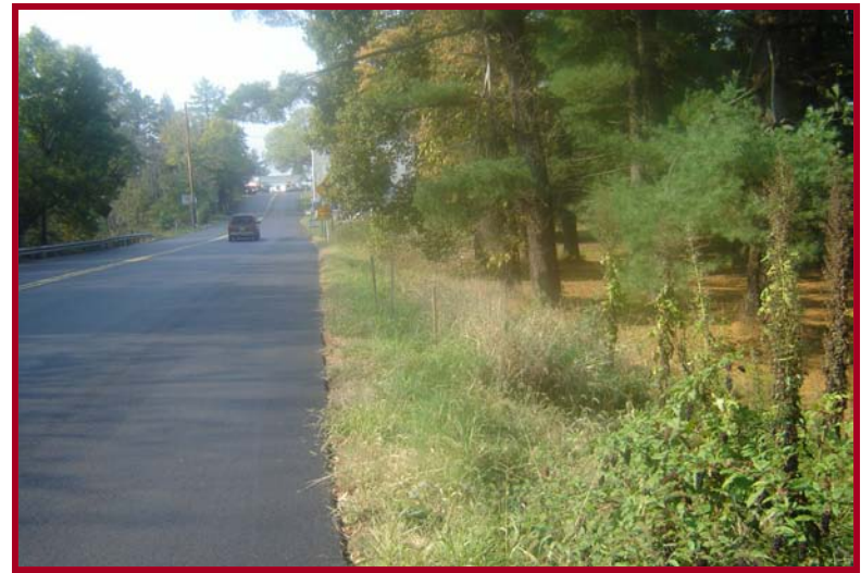
PA 73 (Big Road) looking west prior to bridge – shoulder drop-off
