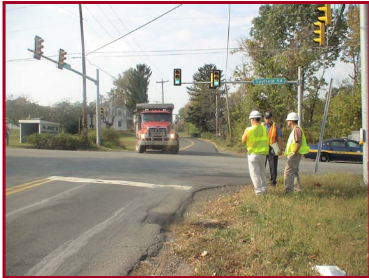
Pavement drop off at the northeast corner of the Hill Road intersection
