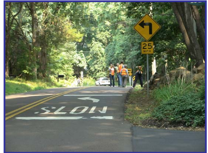
Deteriorating pavement marking on Aquetong Road
