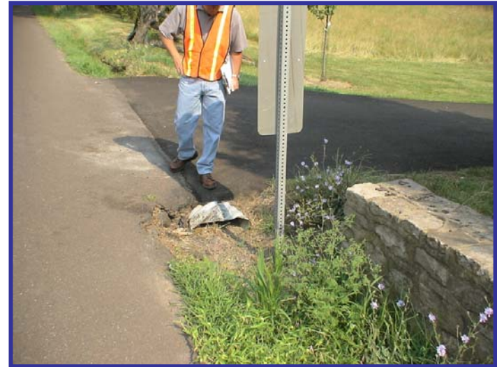
Drain at private property driveway on Aquetong Road west of Cover Bridge Road
