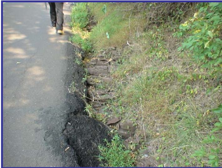
Edge of roadway deterioration on Aquetong Road between Cover Bridge Road and Rockwood Path
