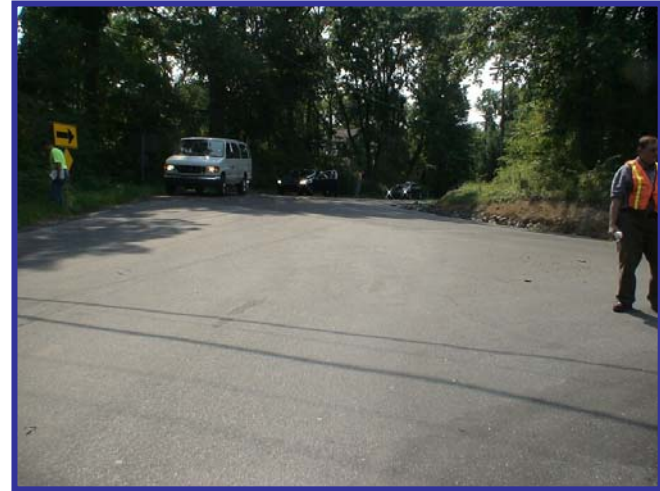
Aquetong Road/Sugan Road intersection Showing no pavement markings
