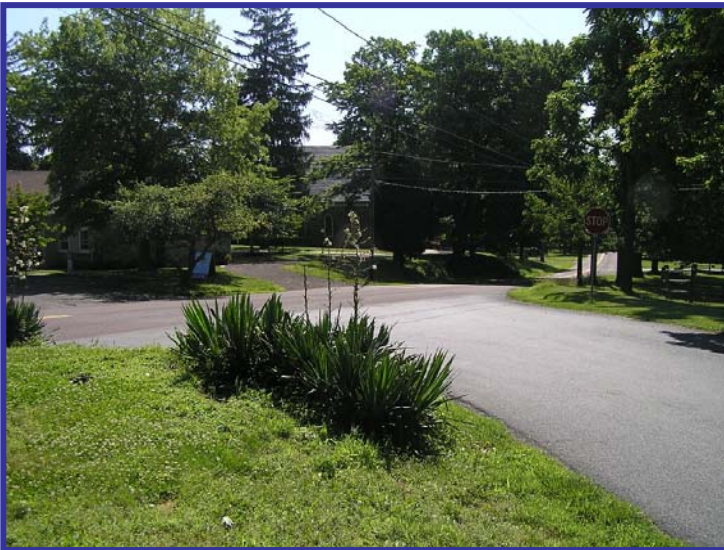
Intersection of Aquetong Road and Cover Bridge Road showing no pavement markings
