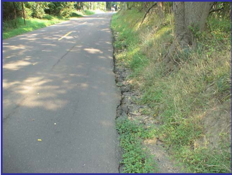
Edge of pavement drop off on Aquetong Road west of Cover Bridge Road
