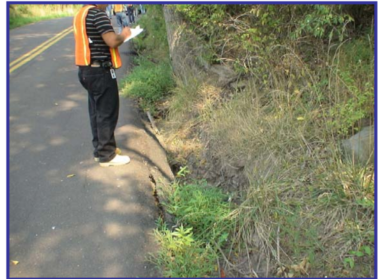
Edge of pavement drop off on Aquetong Road west of Cover Bridge Road
