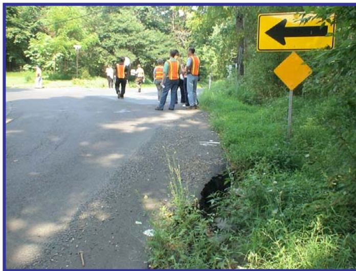
Edge of pavement drop off and deterioration on Aquetong Road east of Sugan Road
