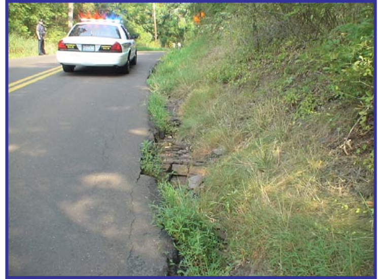
Edge of pavement drop off and deterioration on Aquetong Road west of Cover Bridge Road
