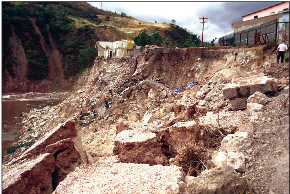
Figure 7. Debris slide at Barrio Mira Mesi adjacent to the Río Choluteca.
