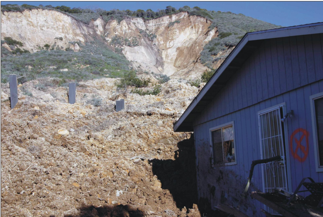
Figure 11. This house was pushed about 3.5 m (12 ft) off its foundation toward the right in the photograph when the 2005 landslide topped a wall. The tops of the H-beams of the wall are visible in the left part of the photograph.
