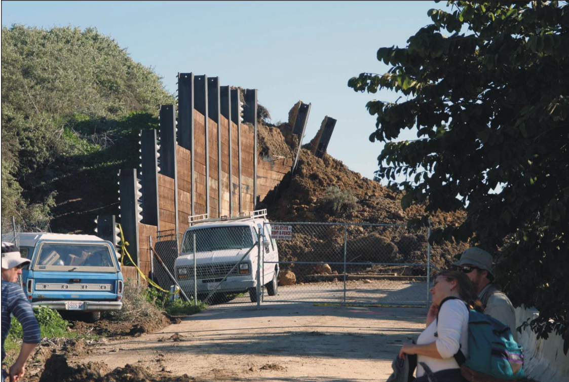
Figure 12. Steel-and-timber wall built after the 1995 landslide was overtopped and tilted forward in places by the 2005 landslide.
