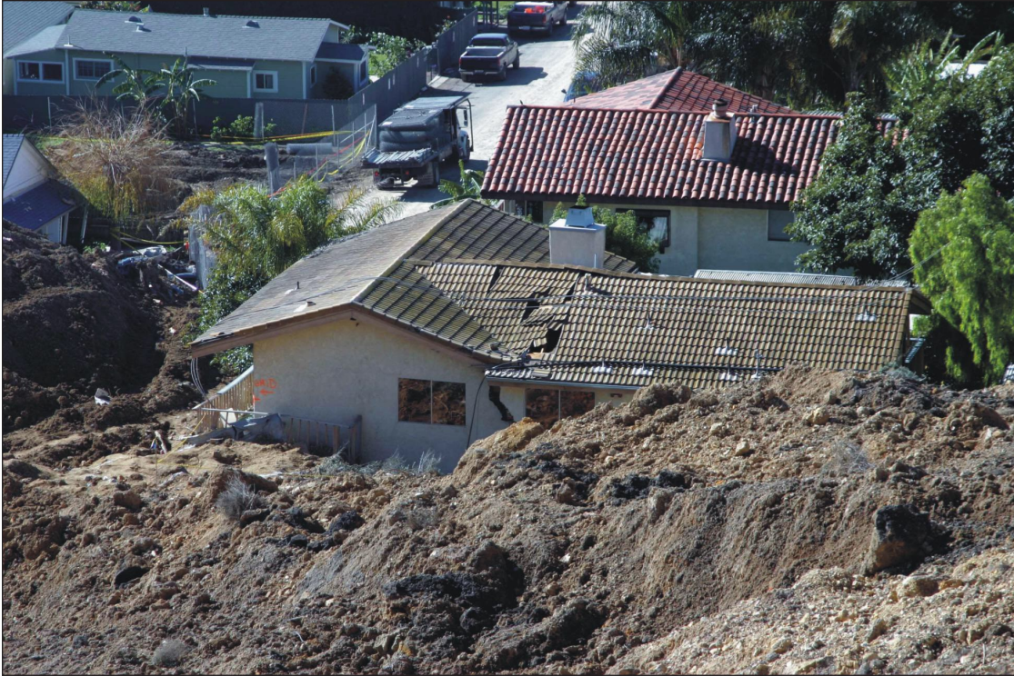
Figure 10. The 2005 landslide moved as a rapid debris flow, but it was quite viscous and pushed houses in its path rather than flowing around or through them. The left part of the house was detached from the right part and was pulled by the landslide several decimeters toward the upper left of the photograph.
