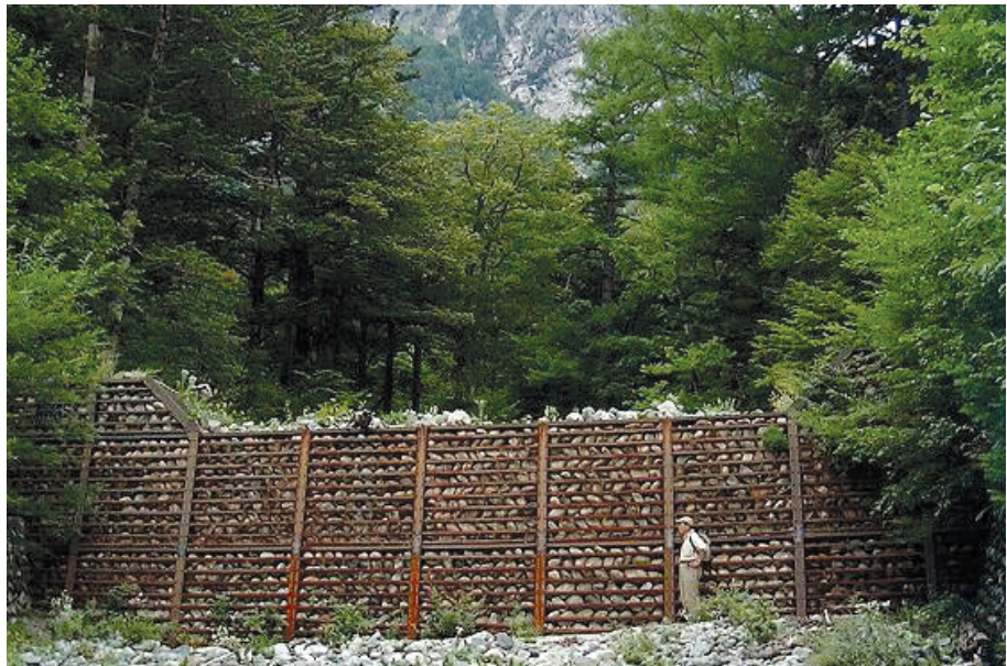
Figure C37. A debris-flow retaining wall in Kamikochi Basin, Japan. (Photograph courtesy of Goncalo Vieira.)
