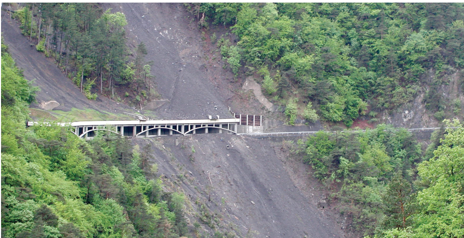
Figure C26. A rock avalanche shelter in the Montenyard area of France. The length of the shelter may be insufficient as a debris flow has damaged the road, shown to the right of the shelter. (Photograph by Dave Giles Engineering Geology Consultancy Group, University of Portsmouth, United Kingdom.)
