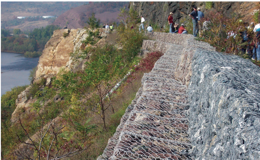
Figure C16. Schematic and photograph of a gabion wall along a highway. (Schematic from Reference 11.) (Photograph of gabions located in the Pocono Mountains, Pennsylvania, USA, by Lynn Highland, U.S. Geological Survey.)
