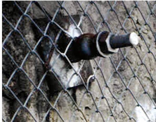
Figure C32. Closeup photograph of a rock anchor on a rock face, with mesh over the surface for more protection. The anchor is set in the rock about 5 meters (15 feet) deep.
