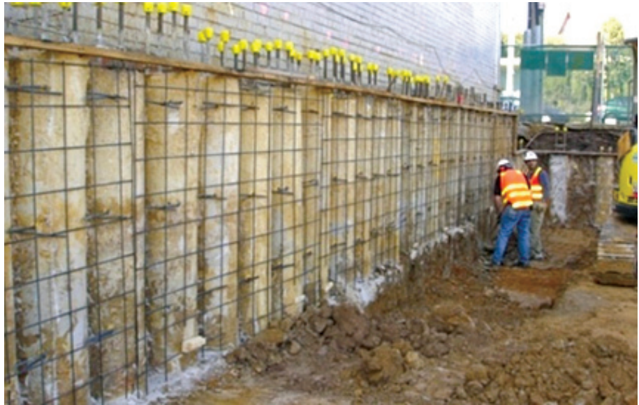
Figure C17. A concrete-filled pile wall. Reinforcing mesh has been hung over face of piles, ready for shotcrete spraying. Location is Brighton, Melbourne, Australia. (Photograph courtesy of Basement Construction Services, Victoria, Australia.)
