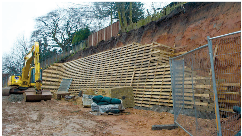
Figure C13. Schematic and photograph of a timber crib. (Schematic from Reference 11, photograph is courtesy of PHI Group, United Kingdom.)
