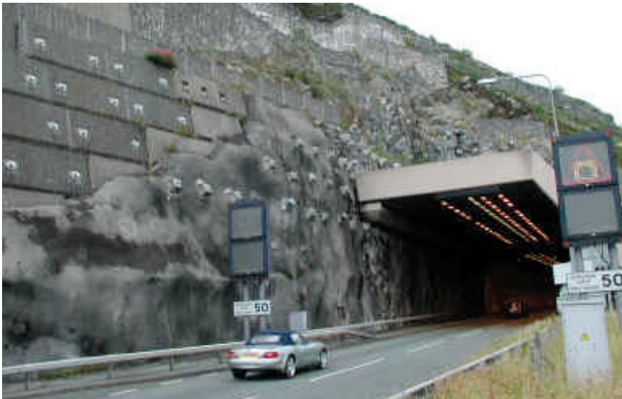
Figure C20. This photograph shows rockfall countermeasures that include mass concrete retaining walls, gabion walls (both wall types are at top of photograph), check fences, boulder treatment, and buttressing. (Photograph is the Pen-y-Clip tunnel on a highway in North Wales, United Kingdom. Photograph by Dave Giles, Engineering Geology Consultancy Group, University of Portsmouth, United Kingdom.)
