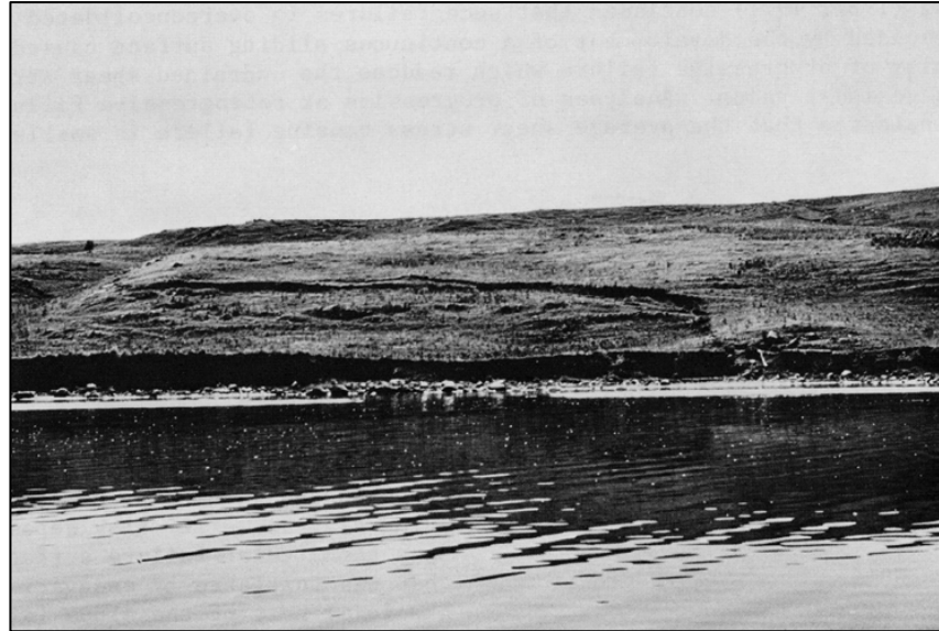
Figure 36. Progressive slump-flow failure of low bluff and adjacent, landward sediments on Lake Ashtabula, ND, apparently initiated by toe erosion at higher water level.
