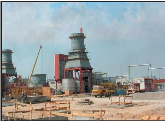
Photograph of new smokestacks under construction at a power plant where USAID funded a project to install two new turbines.
