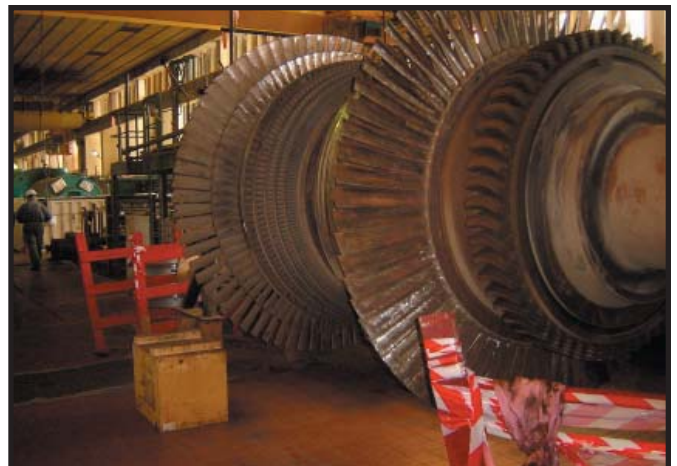
Photograph showing one of two turbines that a USAID contractor refurbished in an Iraq power plant.
