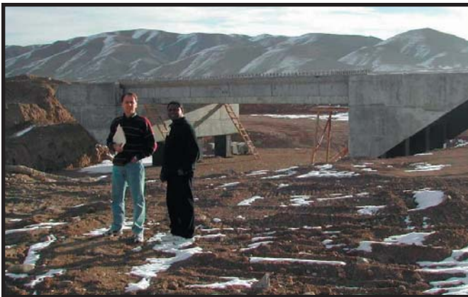
Photograph of RIG/Manila auditors viewing one of six bridges (the first bridge south of Kabul at Km 48) under construction on the Kabul-Kandahar Highway.
