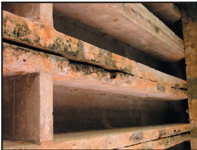
Photograph of concrete beams with corroded steel strands and filtered-down moisture below Los Achiotés bridge in Olancho, Honduras, September 2003.
