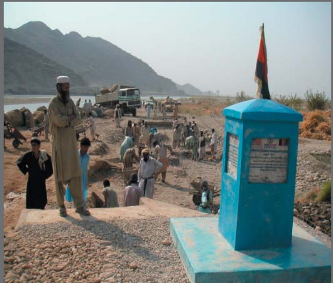
Photograph of Afghan men working on a cash-for-work project to build a flood-protection wall for the village of Binigah, Afghanistan.
