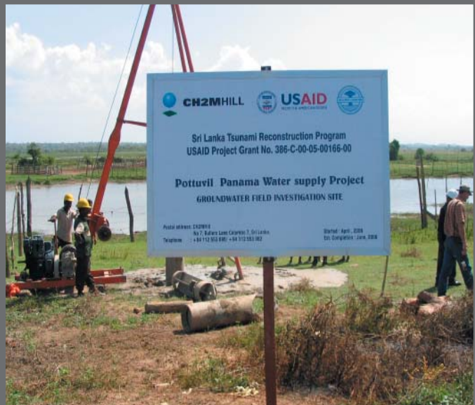
Photograph of drilling operations to determine the feasibility of using groundwater instead of surface water as the water source for the communities of Pottuvil and Panama, Sri Lanka.
