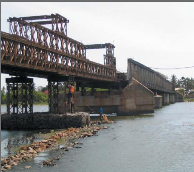
Photograph showing half of the original Arugam Bay Bridge in Sri Lanka that survived the tsunami connected to a temporary bridge. The new bridge will be built adjacent to this bridge.
