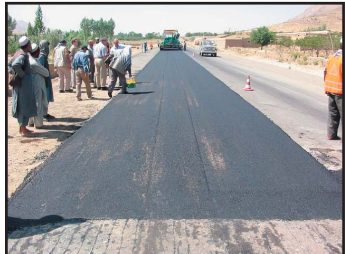
Photograph of construction workers laying asphalt for the Afghanistan highway project between Kabul and Kandahar.
