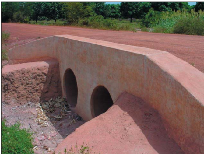
Photograph of a water conduit constructed with Special Self Help Program funds in the Koulikoro region of Mali.
