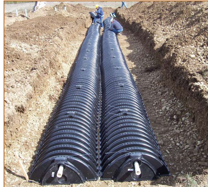
Figure 34: Installation of a pressurized community drainfield for the Martha Boardman community, WA.
