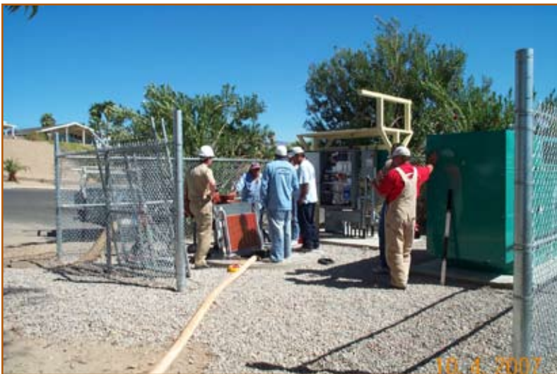
Figure 11: IHS project engineer Roger Hargrove discusses construction with tribal operators and contractors.
