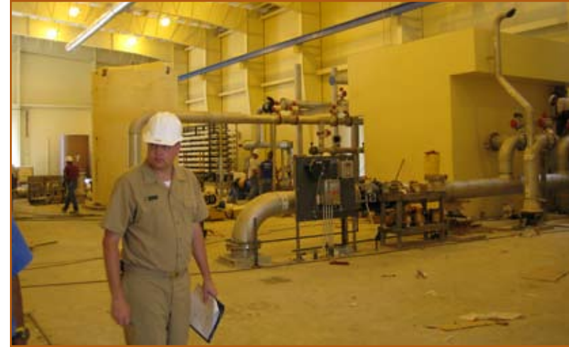
Figure 41: Engineer Scott Helgeson inside the Brighton WTP.
