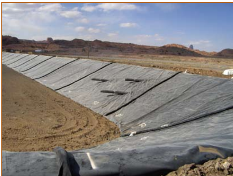
Figure 7: Wastewater treatment lagoon in Kayenta, AZ.
