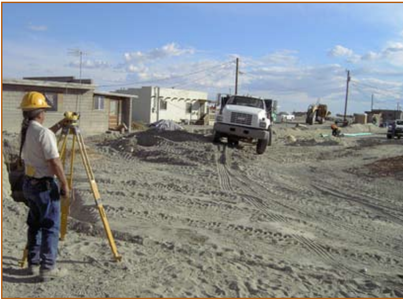
Figure 9: Engineering technician Erwin Tewa shoots grade on the new 8" PVC sewer line extension in Shungopavi Village.
