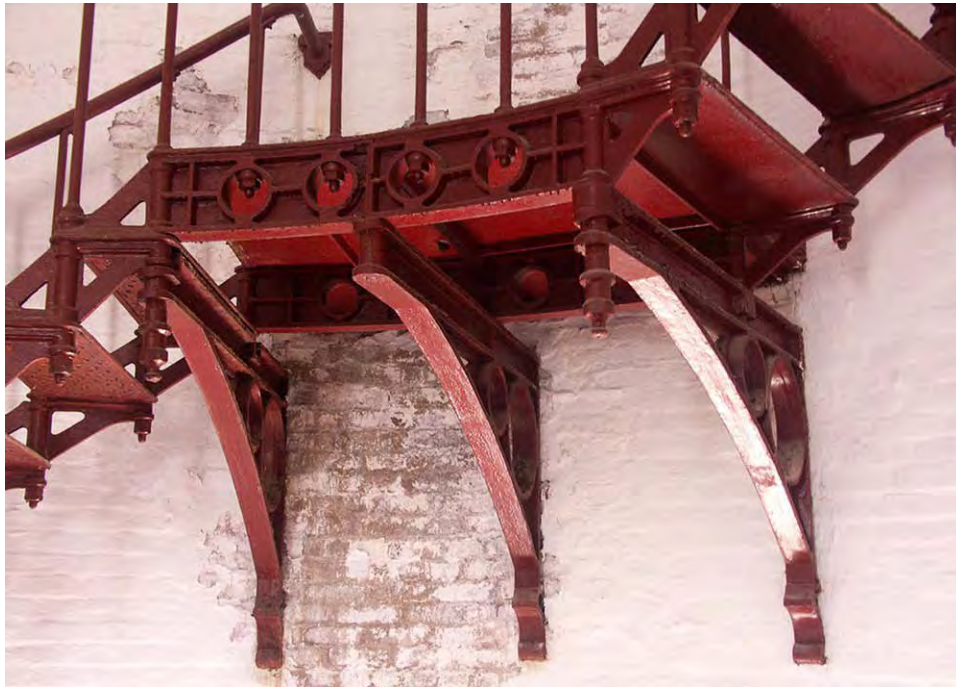
A current photo of the iron circular staircase that lines the inside wall of the lighthouse.
