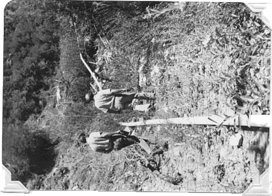
Figure 6. Riparian zone in Water Canyon; bulldozed by Mineop Corp. in order to lay pipe from the water diversion to the mine operations site.
