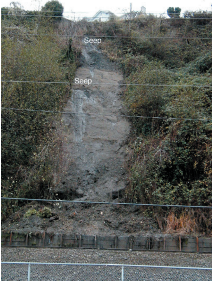
Figure 2. Photograph (view to south, taken December 5, 2001) of landslide that occurred between November 29 and December 5, 2001, about 200 m east of the Everett monitoring site. Rail bed of the BNSF Railway is shown in the foreground. Seeps indicated near east (left) edge of landslide scar are evidence of localized perching and lateral flow of water deeper within the bluff.
