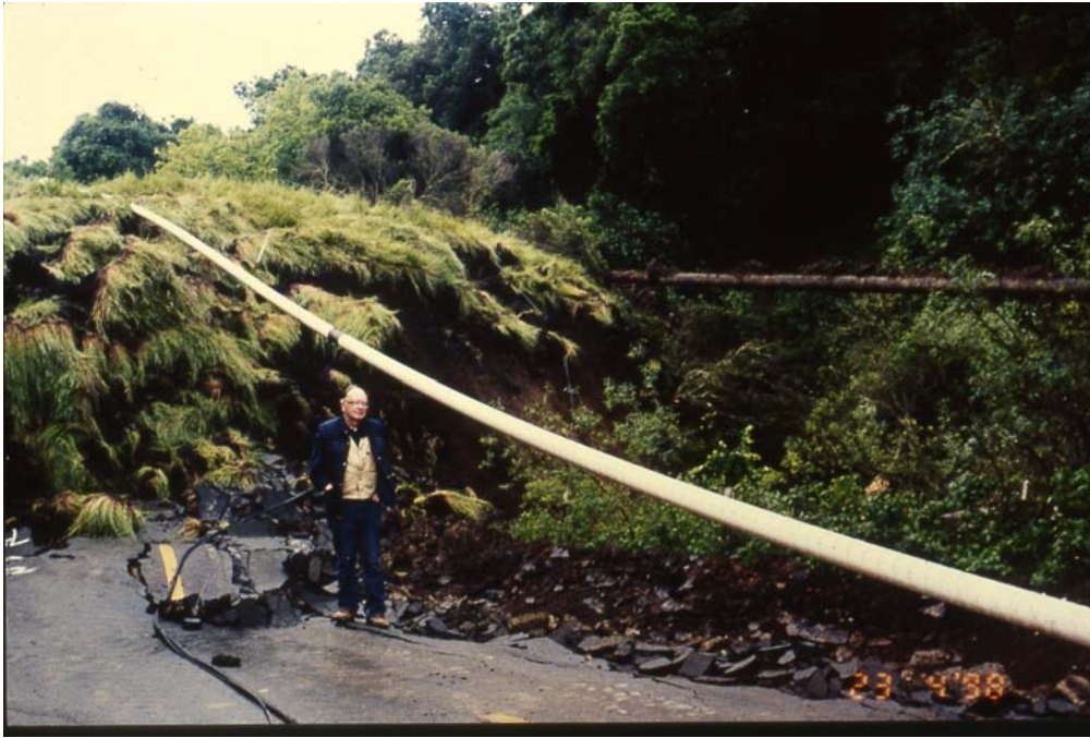
Figure 3-1. Toe of the Anzar Road landslide, San Benito County, California, that severed two 25-cm-diameter gas pipelines on April 22, 1998. The pipelines served approximately 60,000 residential and business customers in Santa Cruz County. The white pipe is a temporary bypass pipe that was placed across the toe soon after the landslide occurred (photograph by Lynn Highland, USGS; Schuster and others, 1998).
