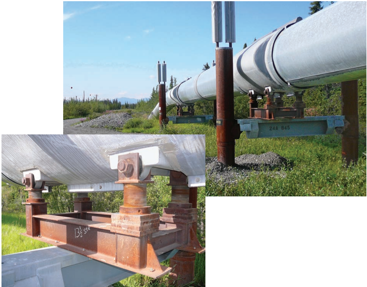
Figure 2.10. Trans-Alaska Pipeline near Glennallen, Alaska (July 2007) showing thermal syphons on vertical support members and adjustable “shoes” to accommodate horizontal and vertical movements. (Photos by Devin Galloway, USGS).
