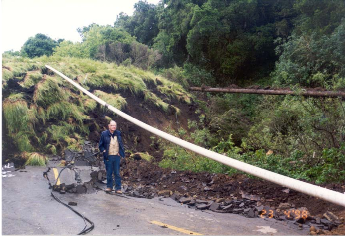
Figure 1B. Toe of landslide in figure 1A showing broken pipeline (brown-colored pipe) and the temporary replacement (white-colored pipe; photo by Lynn Highland, USGS).
