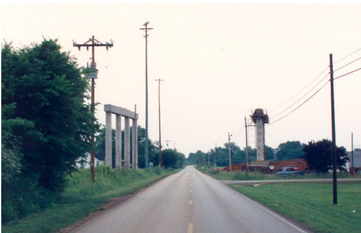
FIGURE 34. The Thompson Lane overpass at the Old Nashville Highway under construction, early 1990s.
