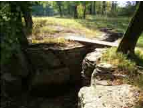
FIGURE 99. Stacked stone alcove containing a spring. Note the wood footbridge that carries the river's edge trail across the alcove.
