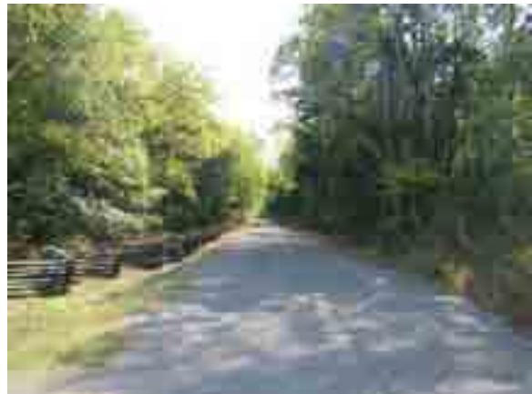
FIGURE 44. Van Cleve Lane as it runs through the Nashville Pike Unit. Note poor road edge conditions.
