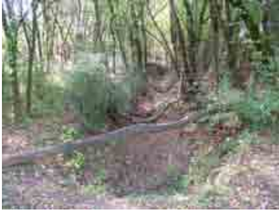
FIGURE 84. Eroded, deeply-channeled ditch near the Stones River Greenway.
