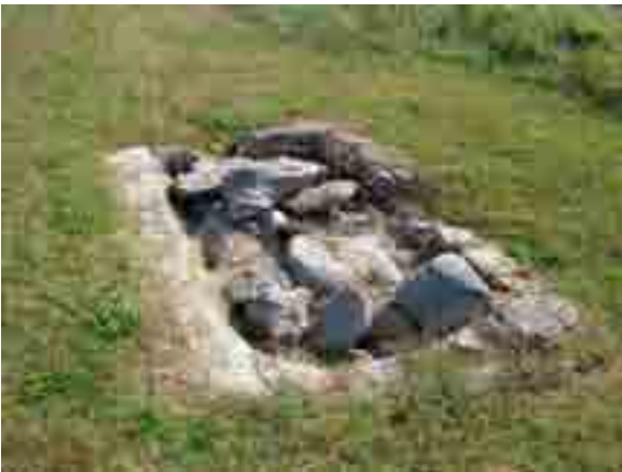
FIGURE 55. Open drainage structure found along the southbound portion of the tour road.
