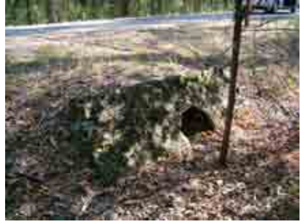
FIGURE 56. Corrugated pipe culvert with a battered stone headwall. Note large amount of organic growth on the stones.
