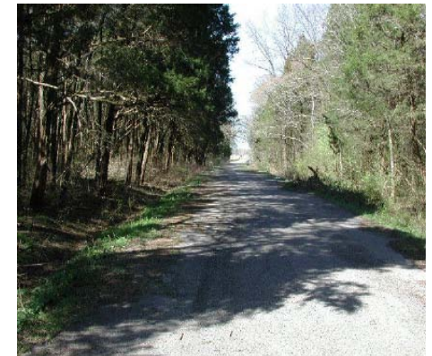
Many of the park roads need repair
