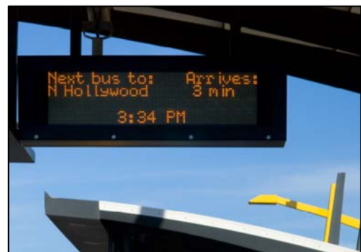
FIGURE 3.8 – Variable Message Sign (VMS)
