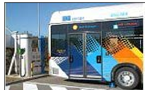
Shell hydrogen refueling station in Luxembourg. Photo courtesy of Shell.
