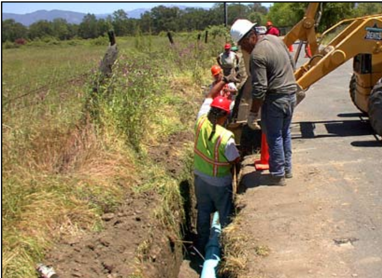
Figure 19: Round Valley's Tribal Force Account crews work diligently to improve water and wastewater services to the reservation.
