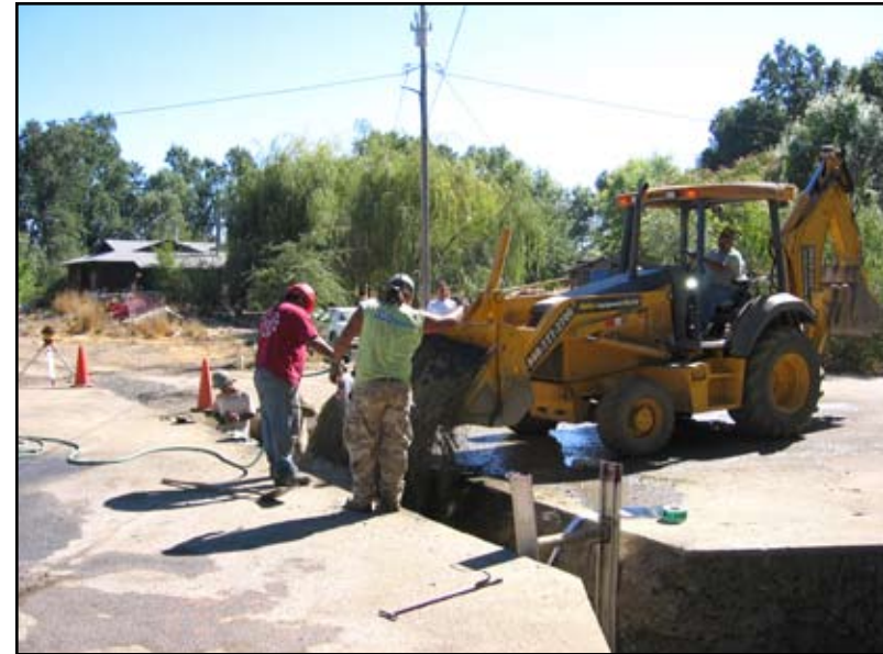
Figure 18: Round Valley's Tribal Force Account crews fill in a trench after installing pipe.
