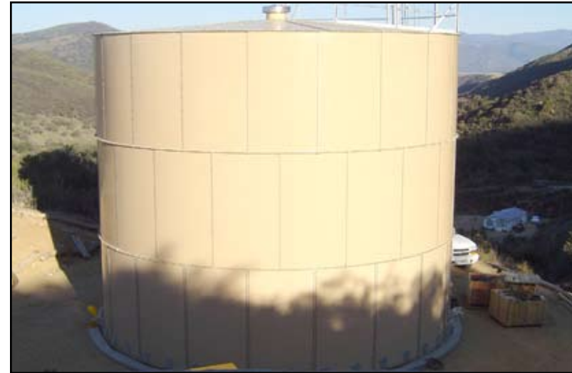
Figure 23: The water storage steel tank.
