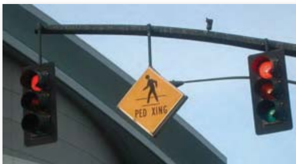
Figure 17. Activated, internally illuminated "PED XING" warning sign hung from a mast arm.
