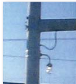
Figure 99. Another detailed view of “rat light.” (Courtesy of the City of Richardson).
