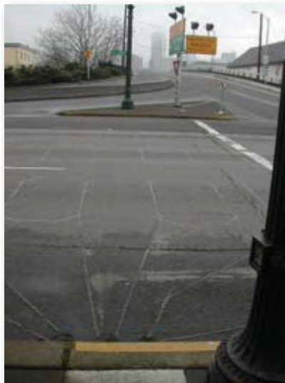
◀ Figure 103 View of inductive loops at stop line for a red light running automated enforcement system in Portland.
