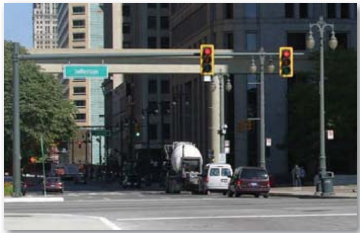
Figure 10. Black signal faces with reflective yellow backplates. (Photo courtesy of Kimberly Lariviere, Michigan DOT).
