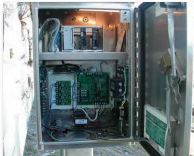
Figure 28. View of inside of the controller cabinet for Florida ramp.
