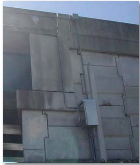
Figure 27. View of pole mounted controller cabinet for in-pavement speed reduction system mounted on an elevated ramp above.
