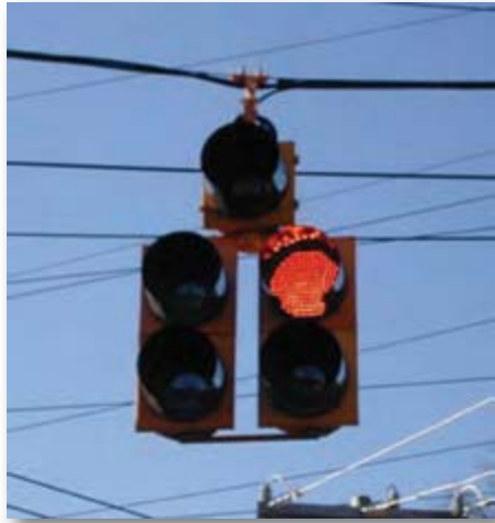
Figure 9. Signal head with LED sections.
