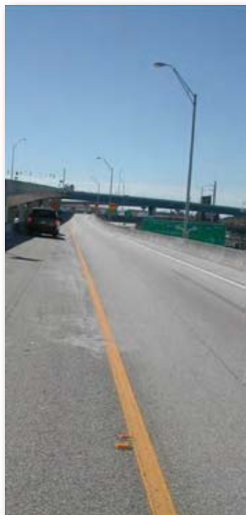
◀ Figure 29. View of in-pavement lighting device and sealant showing sawcut for cable.
