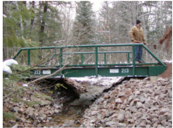
One of several new, clear-span bridges that control erosion and allow fish migration Photograph by Joe Wagner
