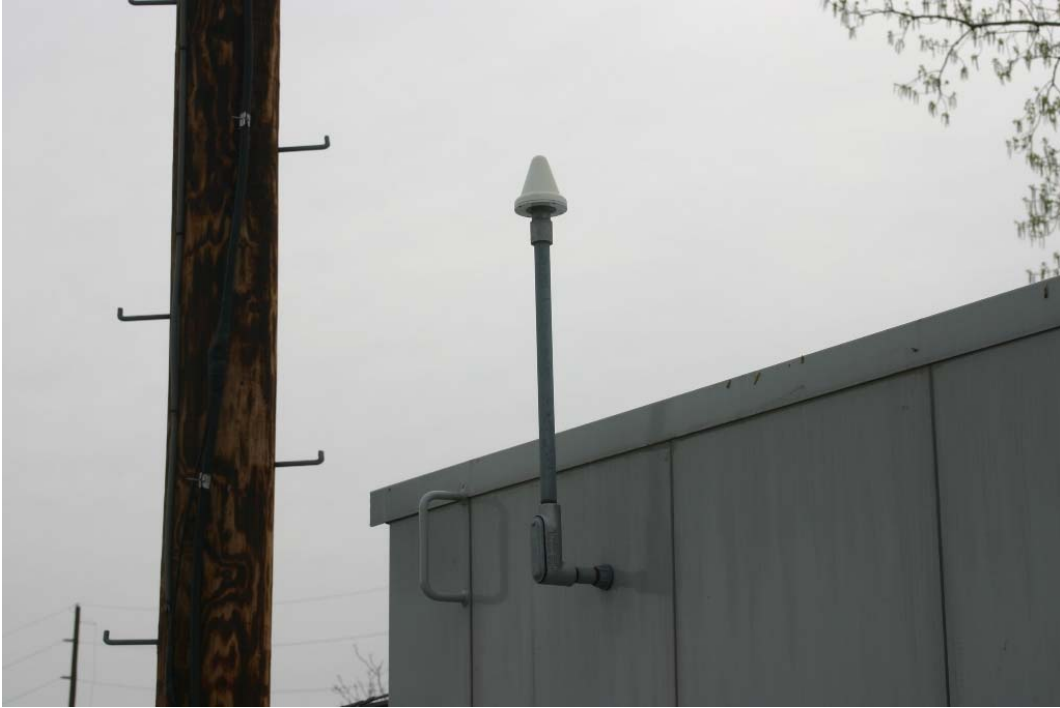
Figure A-8. Typical GPS Antenna Installation on WIU Housing
