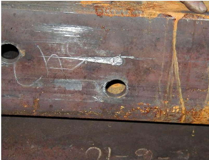
Figure 5. Bolt Hole in the Sliding Sill of One of the Crush Zones After the Test
