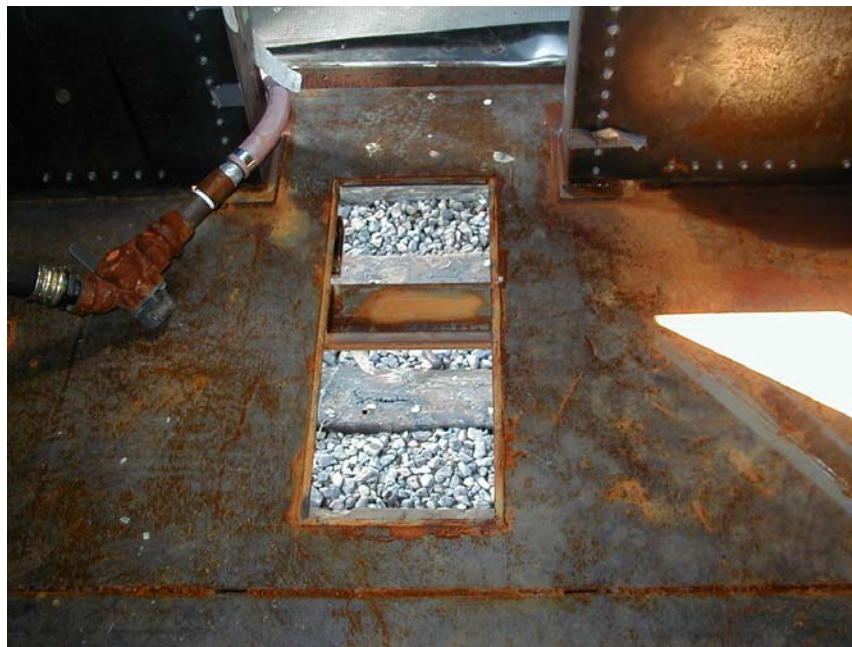
Figure 15. Access Hole Cut in the Floor Plate in the Vicinity of the Sliding Sill/Fixed Sill Connection
