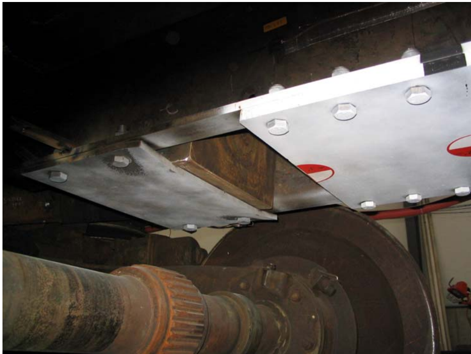
Figure 7. Cover Plate on the Bottom of the Sliding Sill Immediately Below the Buff Lug
