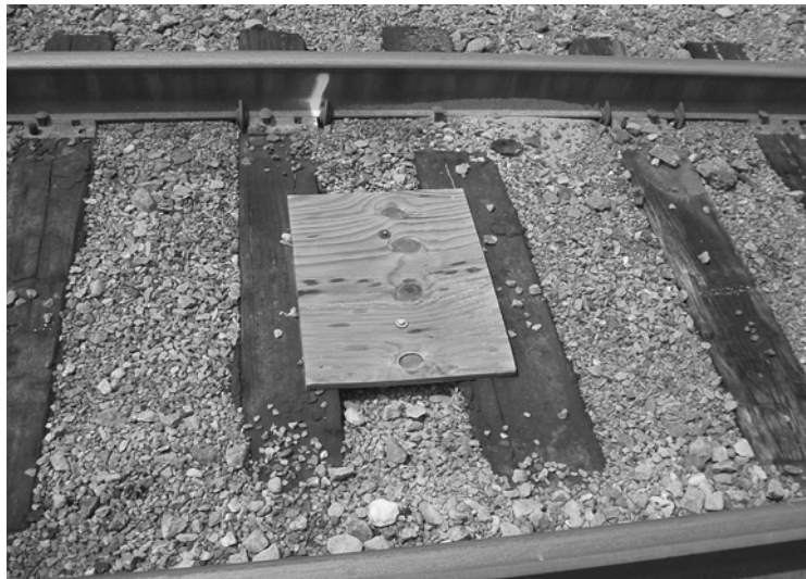
Figure 33. RCL3 stop transponder embedded under plywood in east lead track
