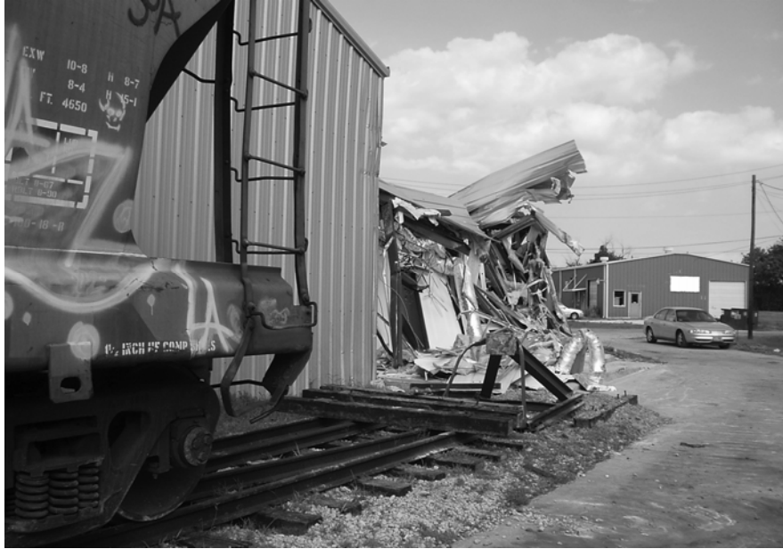
Figure 52. RCL5 damaged bumper post and industry building conference room
