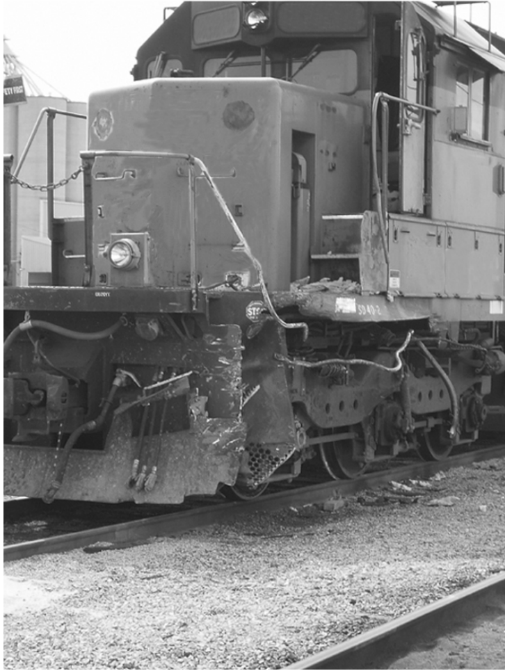
Figure 16. RCL1 damaged 111 RCL
