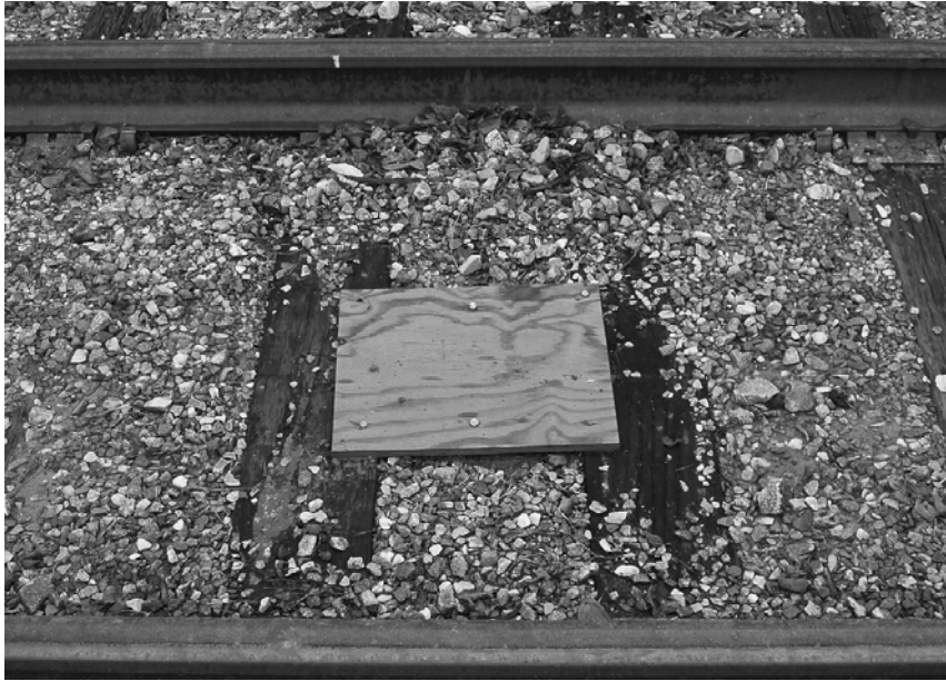
Figure 57. RCL6 automatic pullback protection system transponder mounted under plywood (visible) and embedded in track
