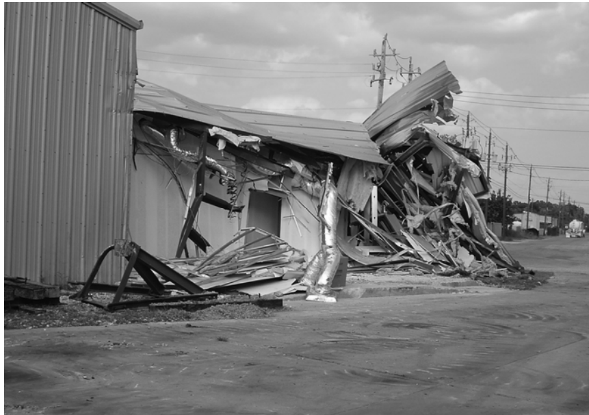
Figure 53. RCL5 damaged industry building conference room
