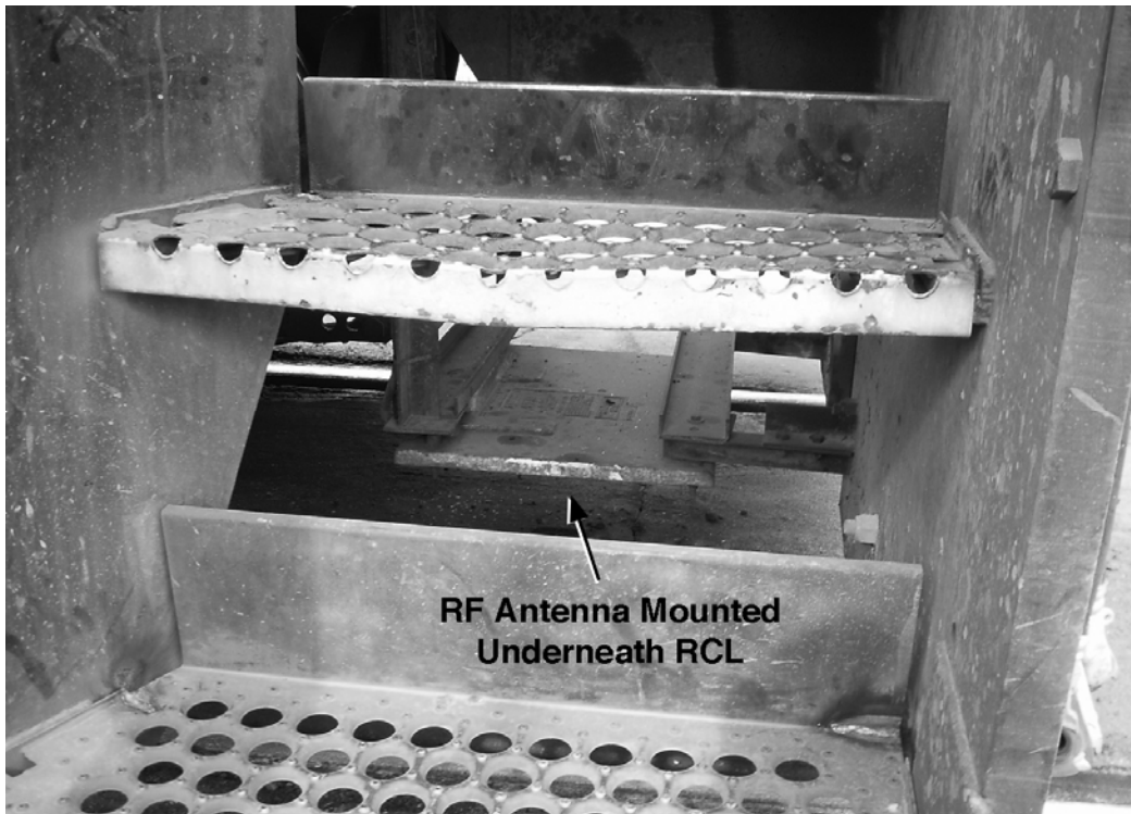
Figure 59. RCL6 pullback protection system RF antenna mounted beneath locomotive
