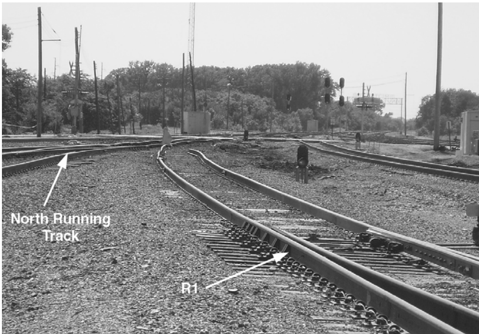
Figure 22. RCL2 location of collision and damaged track (out of service indicated by flag on left rail)
