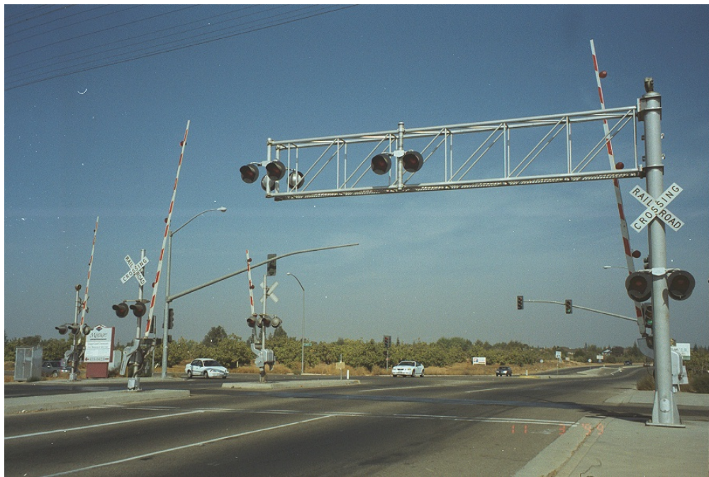
Figure 3. Public Crossing with Flashing Lights, Gates, and Traffic Signals
