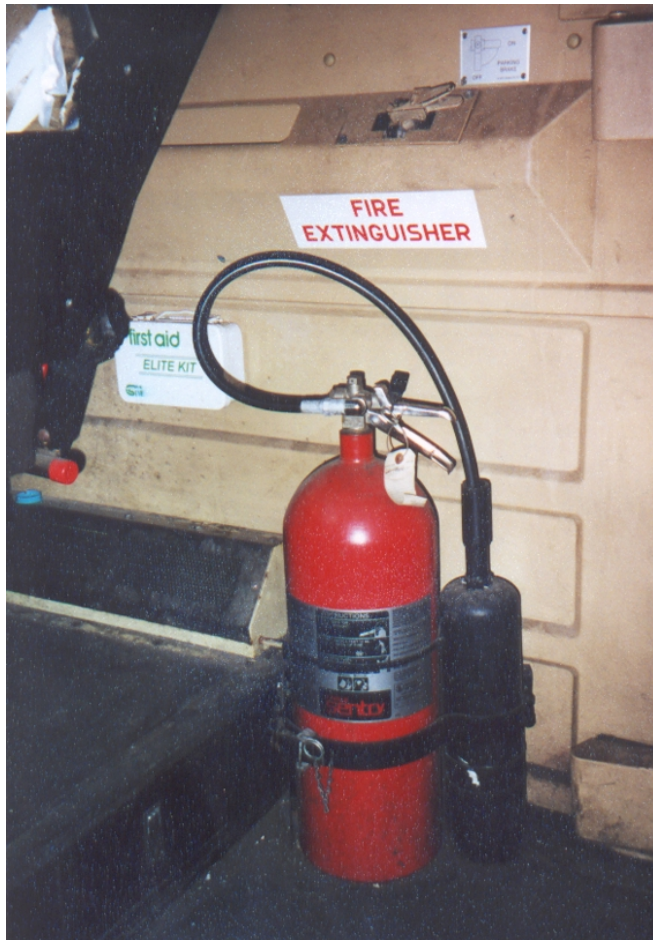
Figure 109. P32-AC fire extinguisher located immediately behind engineer's seat
