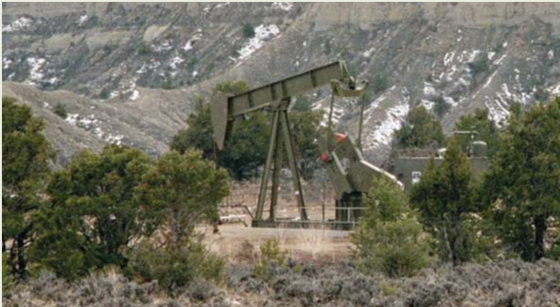
This pumping unit has been painted a color that helps it blend in with the surrounding juniper tree screening.
