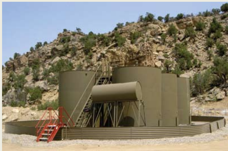
This central tank battery has been surrounded with a corrugated metal containment wall.
