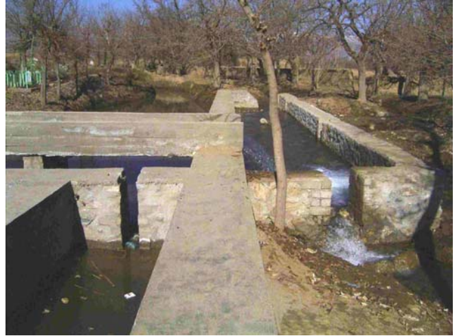
Photograph of improvements made to Charikar Canal after rehabilitation (RIG/Manila auditor took the photograph in December 2005).
