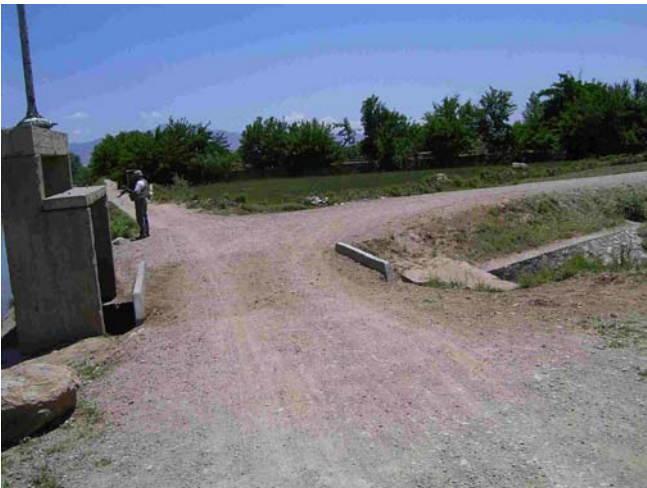
Photograph of a bridge structure on the Canal Road in the province of Parwan, Afghanistan after rehabilitation (RIG/Manila auditor took the photograph in May 2005).
