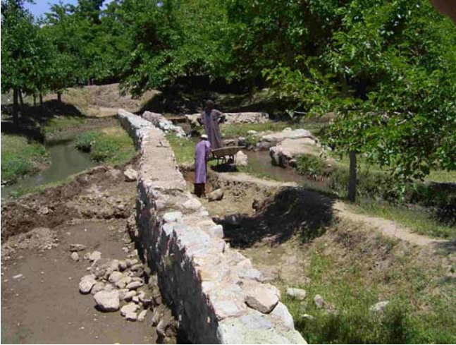
Photograph of the Charikar Canal's Five-Fingers Extension structure in the province of Parwan, Afghanistan before rehabilitation (RIG/Manila auditor took the photograph in May 2005).
