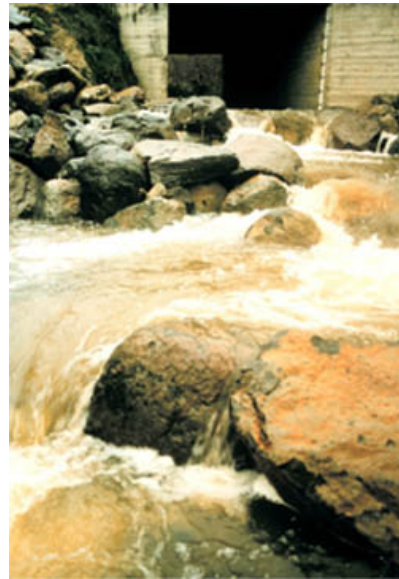
Step pool fish passage provides salmon and trout access through a culvert to upstream spawning grounds
