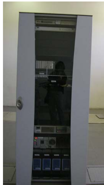
Photo of a signal rack at a power plant. (Central Iraq - September 2006)
