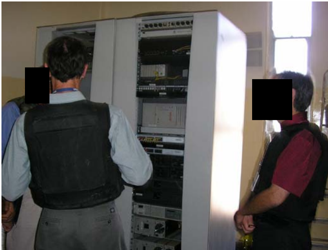
Photo of consolidated fiber network equipment at a power plant. The tower on the left is the operator. The tower on the right is the data receiver. (Central Iraq - September 2006)
