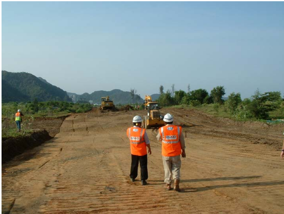
OIG photograph of road construction near the Raba River bridge crossing at Km 25 in Aceh Province, Indonesia. (March 2007)
