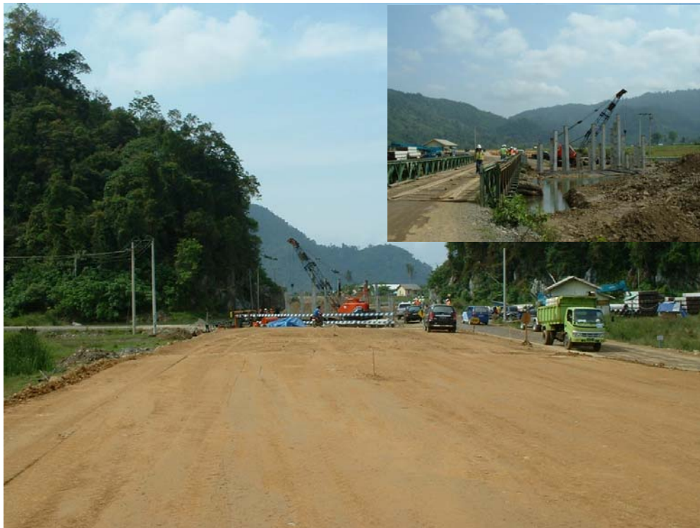
OIG photograph of road and bridge construction at Km 46 adjacent to existing road with green dump truck on it (right side) in Aceh Province, Indonesia. Inset: opposite view of bridge construction (right side) next to a temporary bridge (left side). (March 2007)
