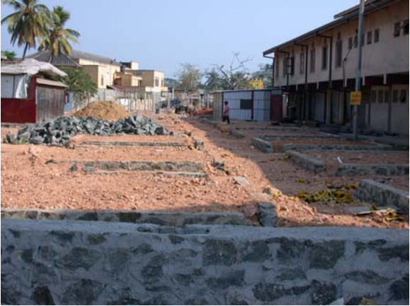
OIG photograph of the Kotuwagoda market under construction with the stalls clearly demarcated by concrete slabs. The construction of the market is funded by USAID under the tsunami supplemental fund. (Matara, Sri Lanka, March 2007)
