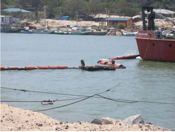
OIG photograph of the USAID-funded sand-conveying pipes attached to the dredging machine and used in dredging sand from the mouth of the Kirinda harbor. (Hambantota, Sri Lanka, March 2007)
