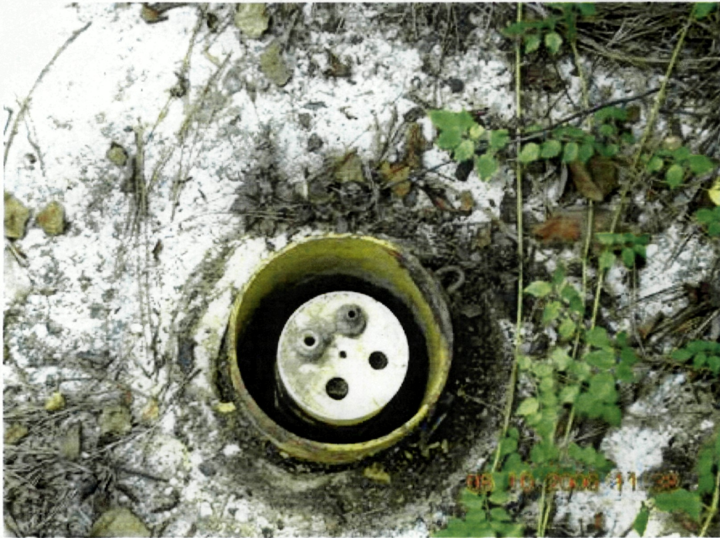
Photo 36: View inside outer protective casing at monitor well GW-23. A dust cap is missing from the well cap.
