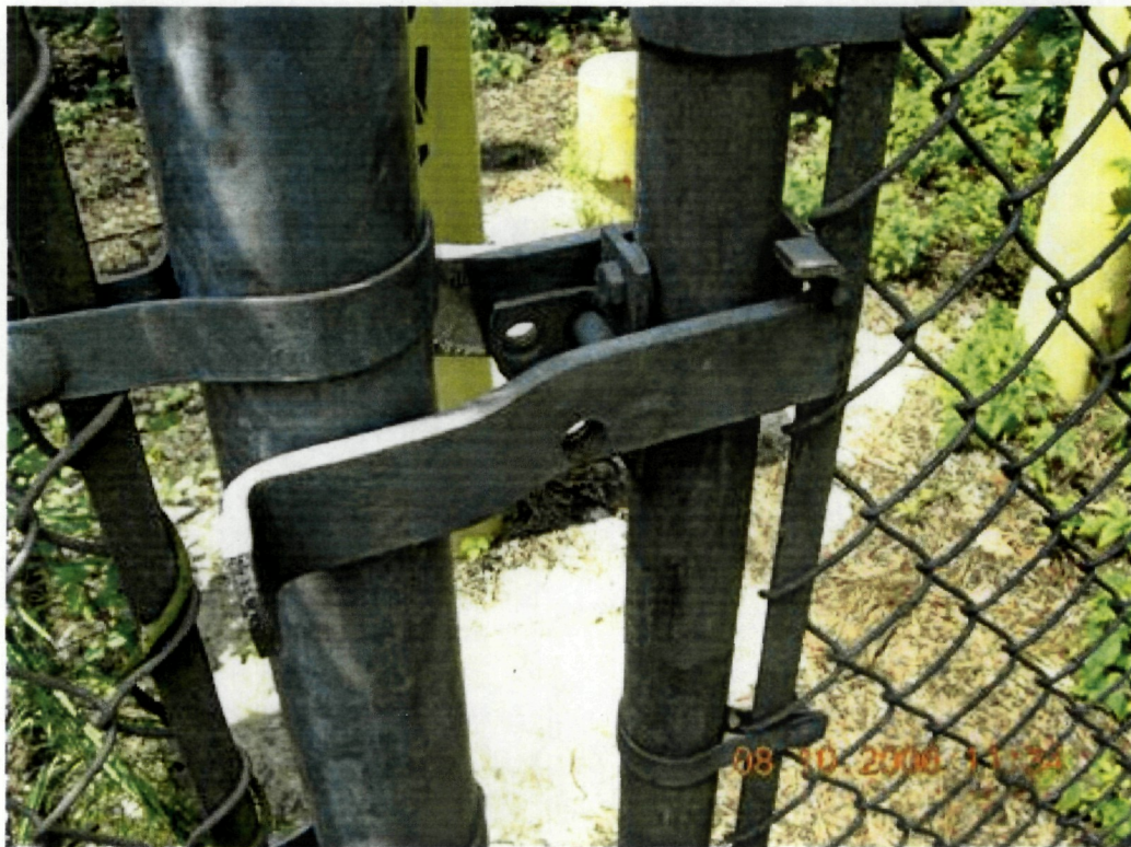
Photo 32: Missing gate lock at monitor well GW-07.
