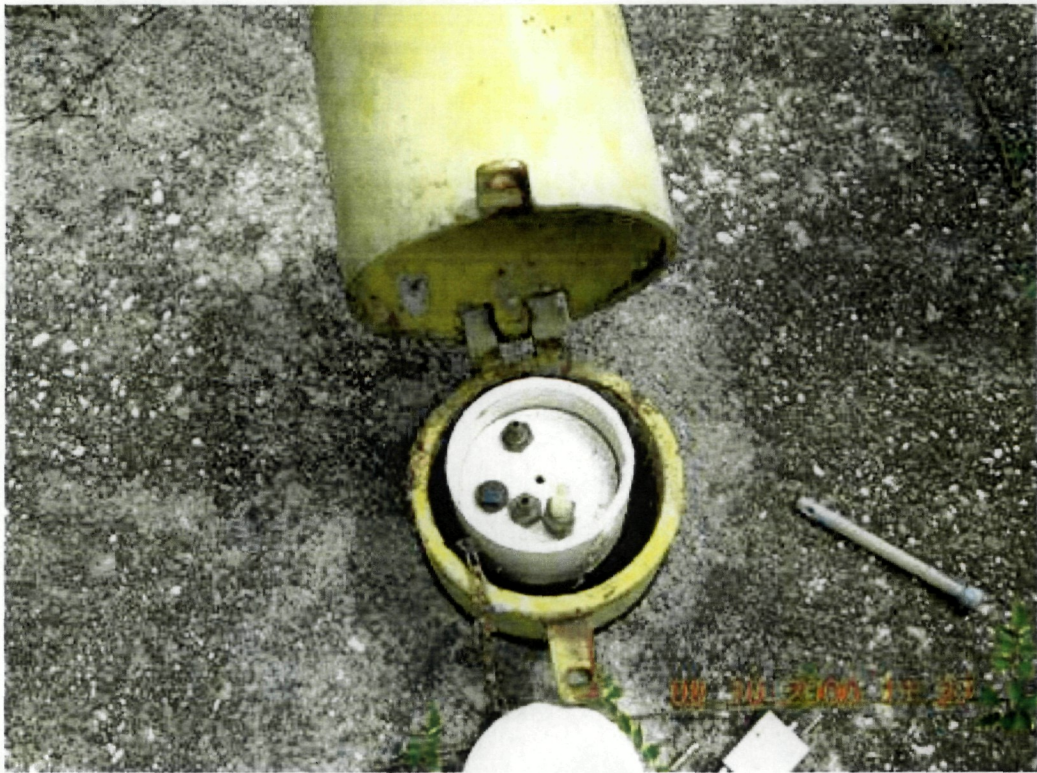
Photo 28: View inside outer protective casing at monitor well GW-21.
