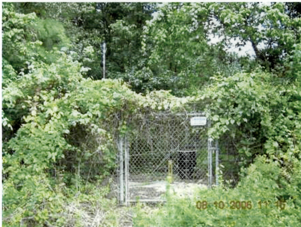
Photo 19: View of monitor well GW-35. Chain link fence is properly secured. A single drum is stored inside the fence.
