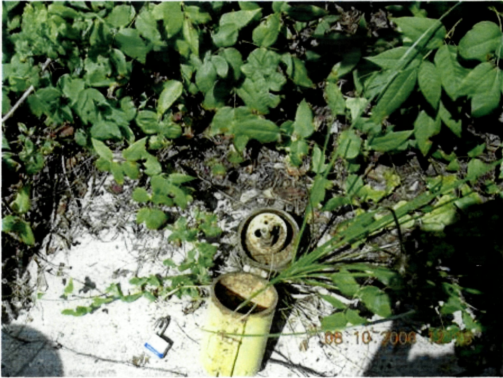
Photo 55: View inside outer protective casing at monitor well GW-15. A dust cap is missing from the well cap.
