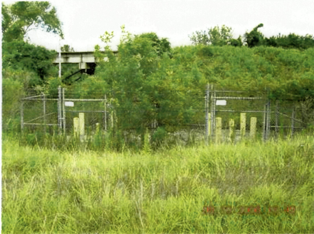
Photo 12: View of chain link fence at monitor well GW-32 and GW-33 facing northwest. Warning sign is still posted (it is behind the tree) and in good condition.
