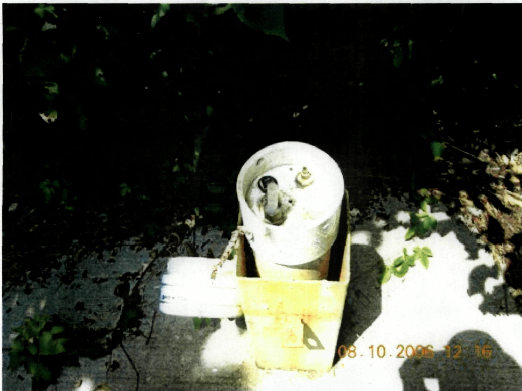
Photo 54: View inside outer protective casing at monitor well GW-31.
