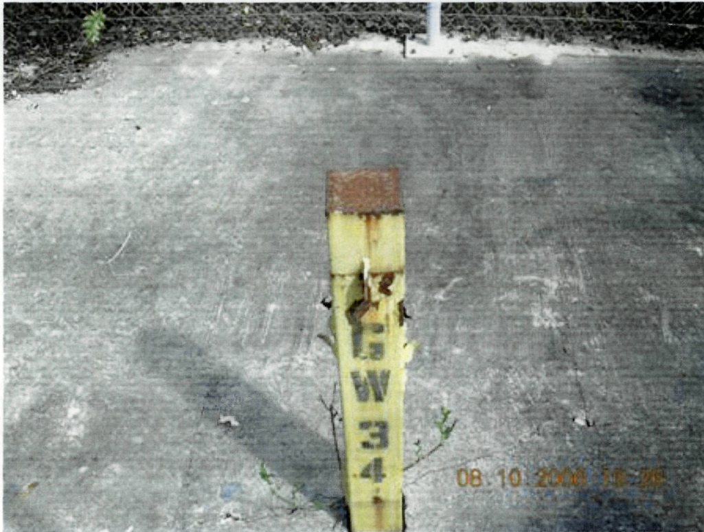
Photo 3: The lock is missing on the outer protective casing at GW-34.
