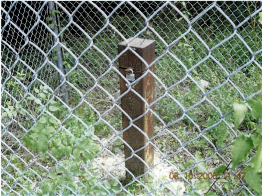
Photo 39: View of monitor well INT-116. The outer casing is properly secured.
