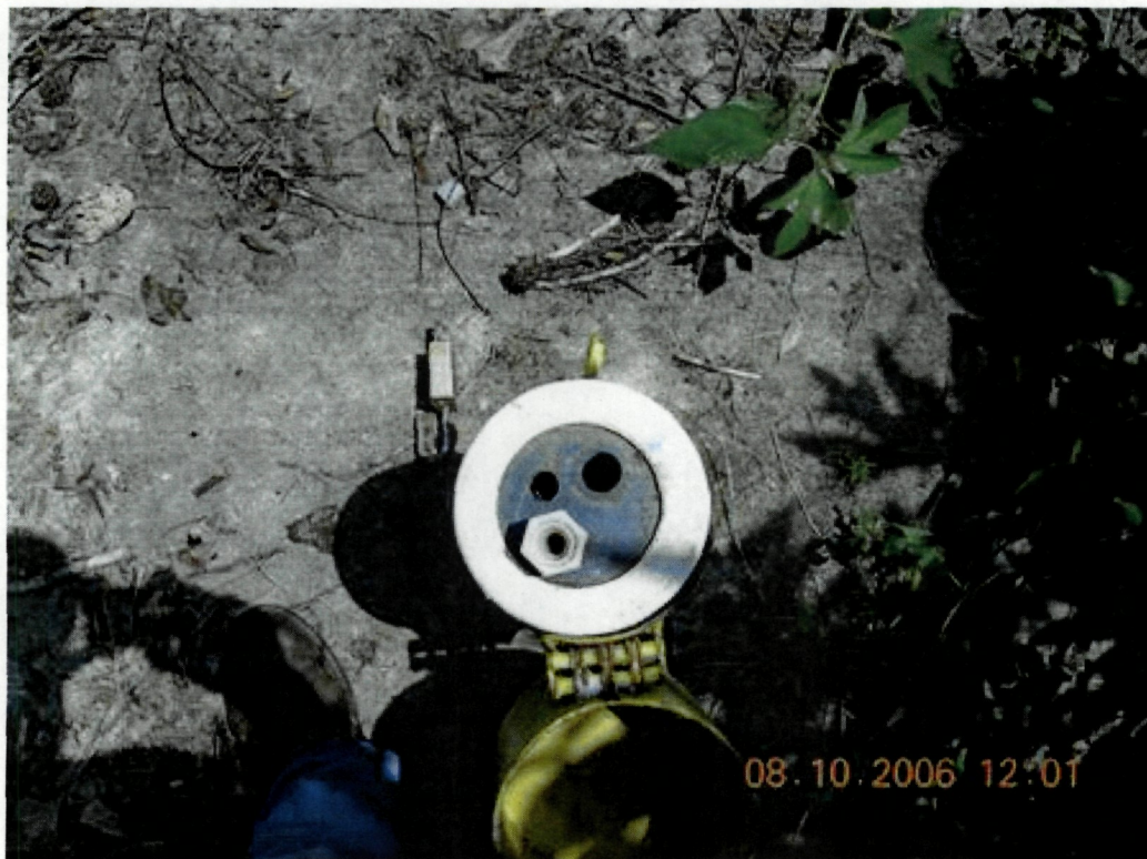
Photo 45: View inside outer protective casing at monitor well GW-25. A dust cap is missing from the well cap.
