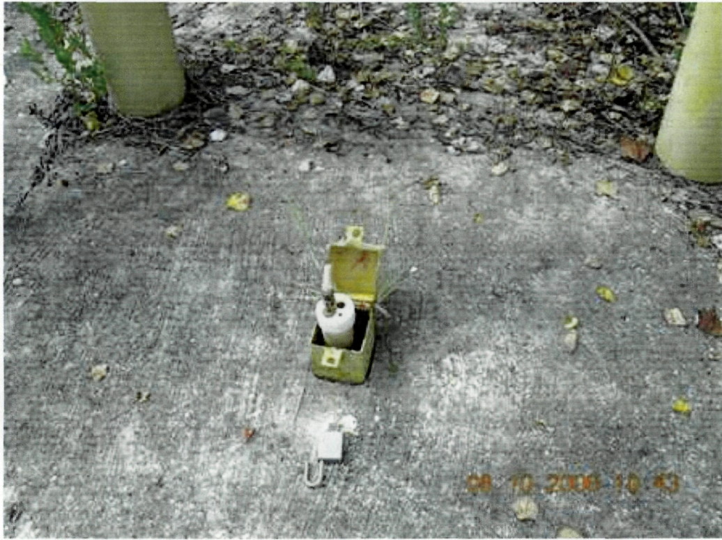
Photo 11: View inside outer protective casing at monitor well GW-28. A dust cap is missing from the well cap.
