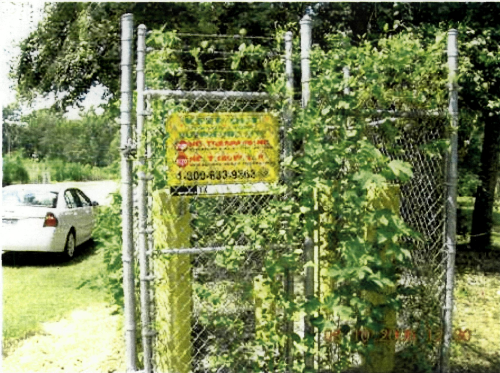
Photo 44: View of chain link fence at monitor well GW-25. Warning sign is visible and in good condition.
