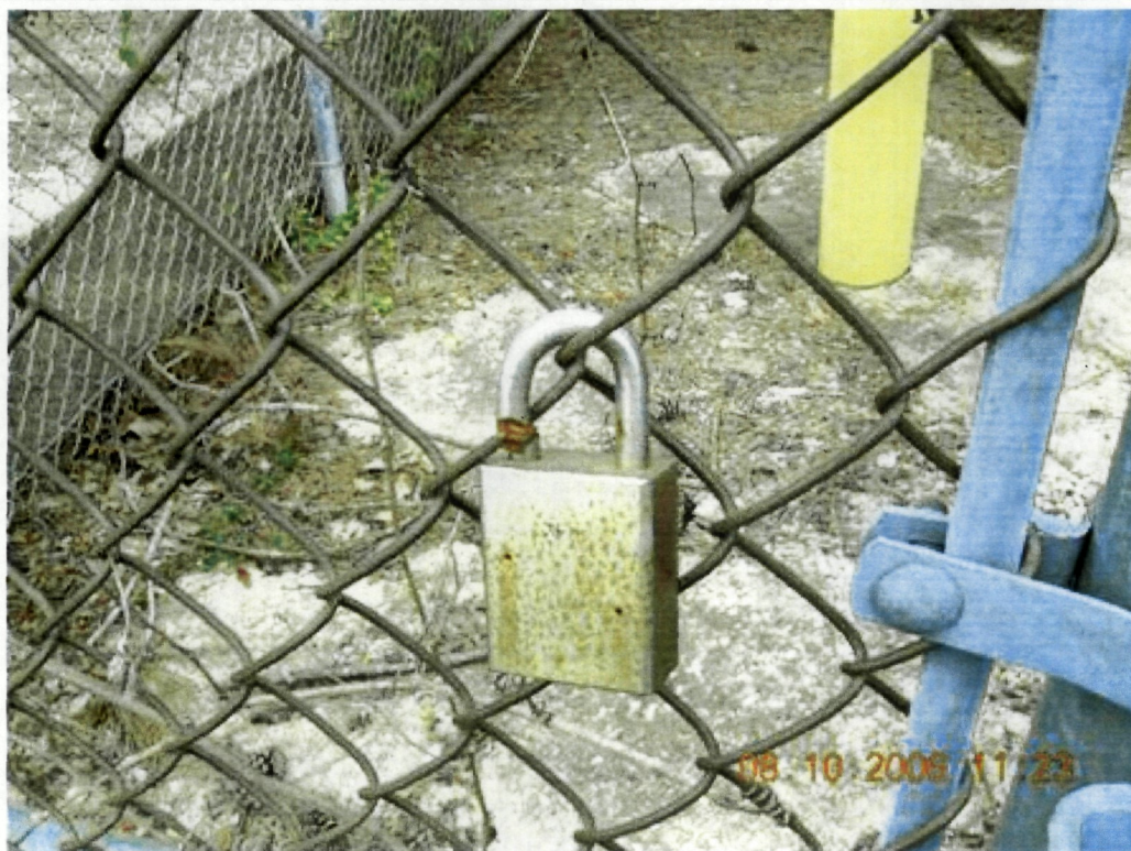
Photo 24: Broken lock on chain link fence at GW-27
