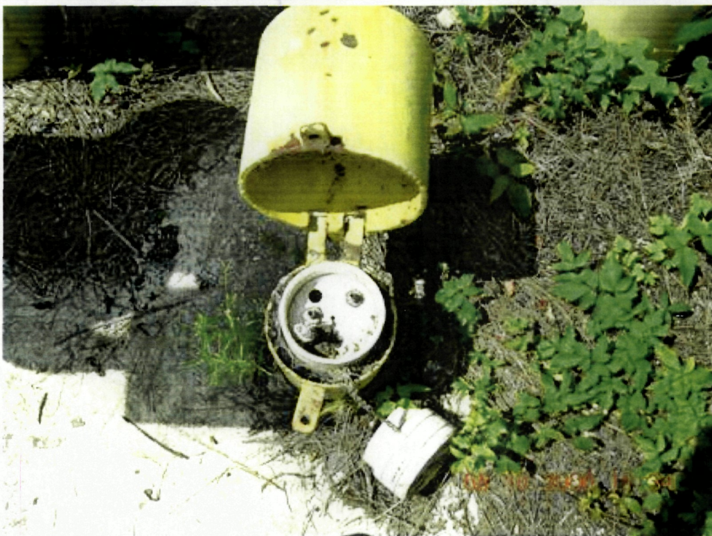
Photo 30: View inside outer protective casing at monitor well GW-07. A dust cap is missing from the well cap.
