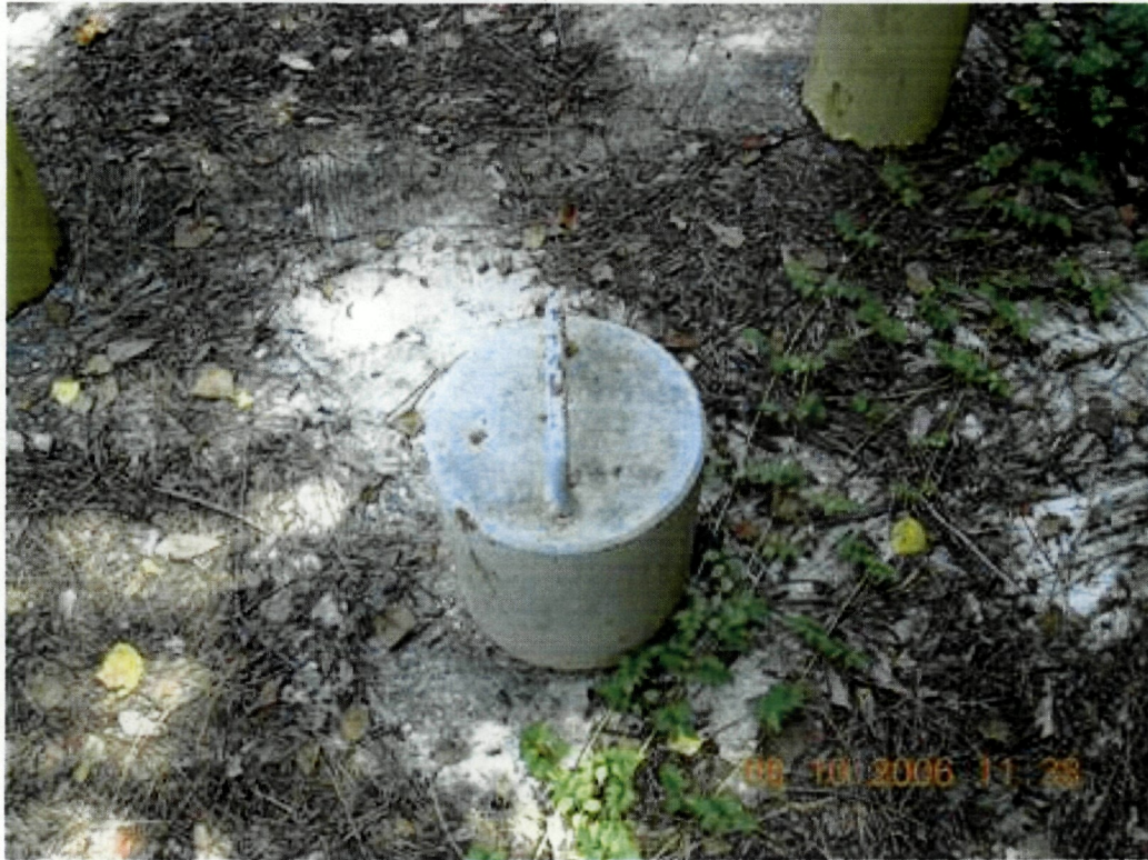
Photo 35: View of outer protecting casing at GW-23. The casing does not have a securing mechanism.
