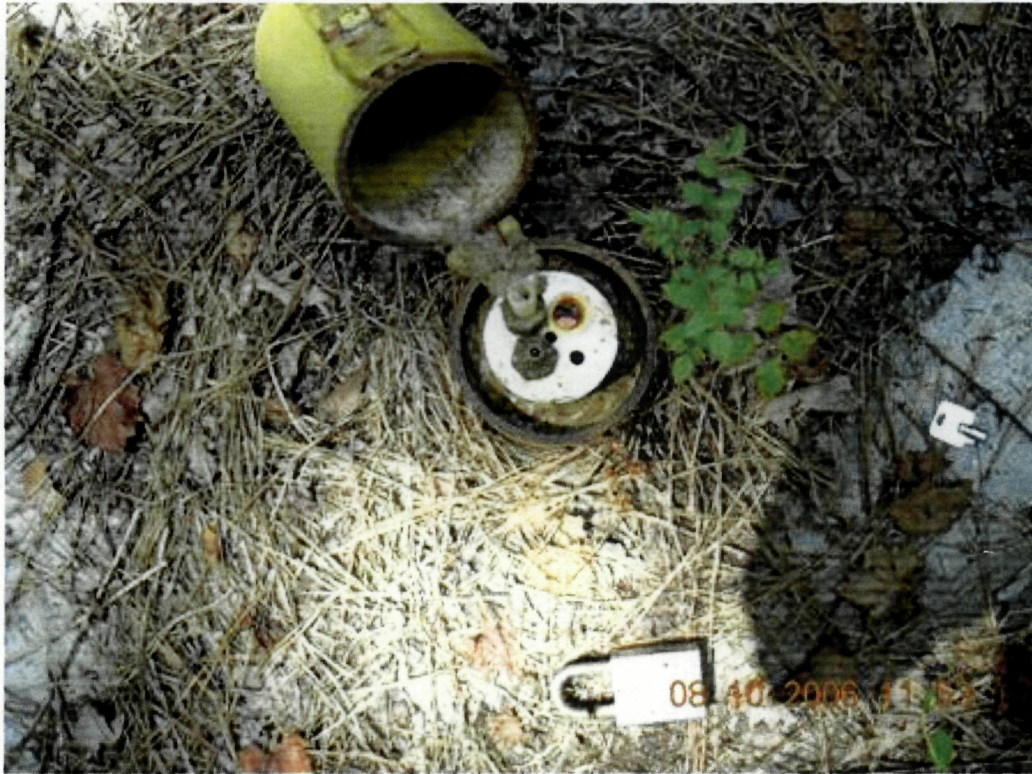
Photo 43: View inside outer protective casing at monitor well GW-19.
