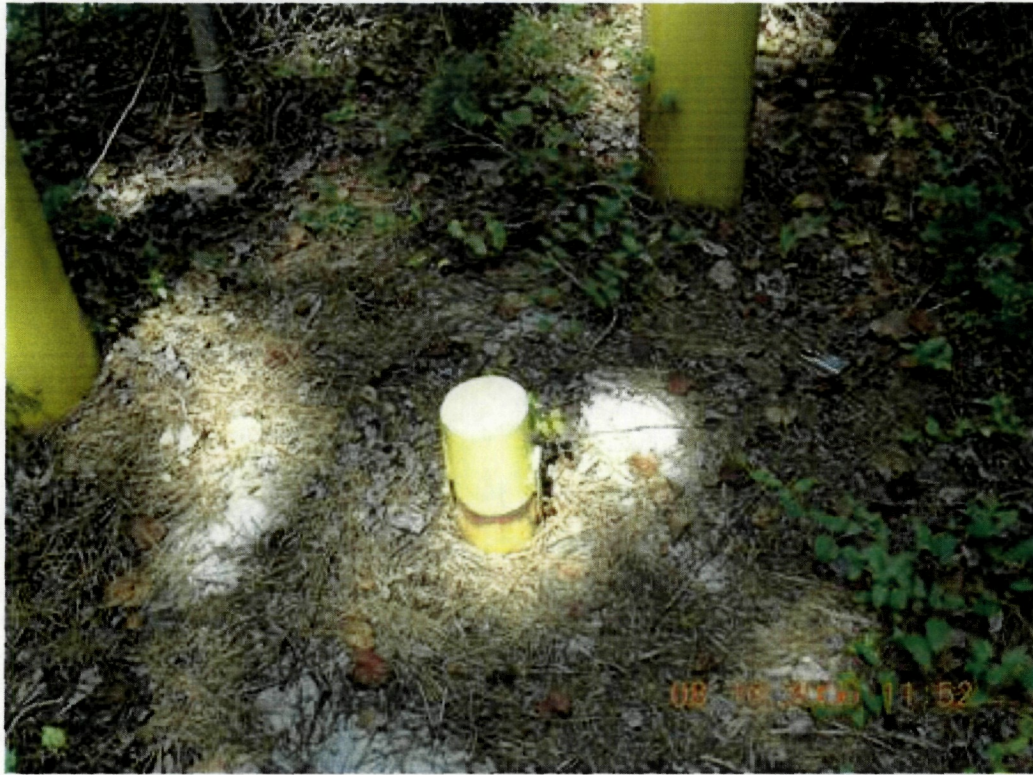
Photo 41: View of protective casing at monitor well GW-19.
