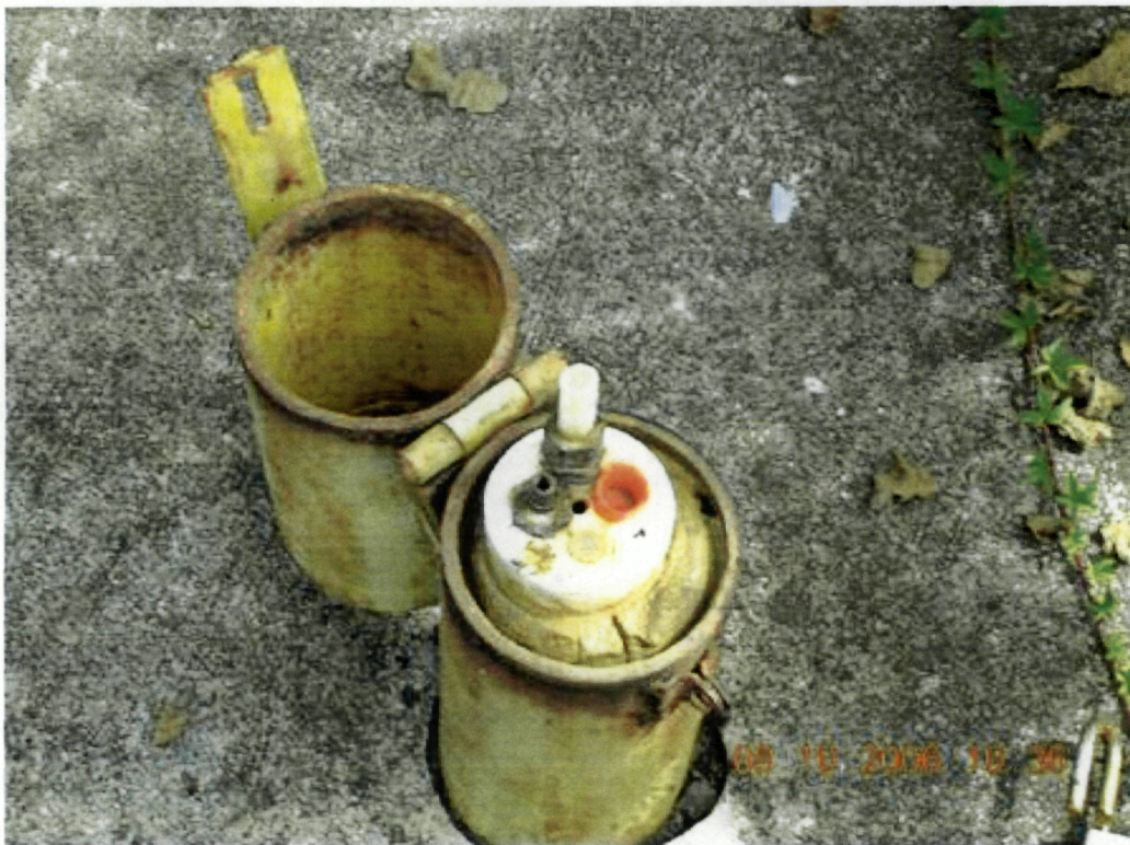
Photo 6: View inside outer protective casing at monitor well GW-18.
