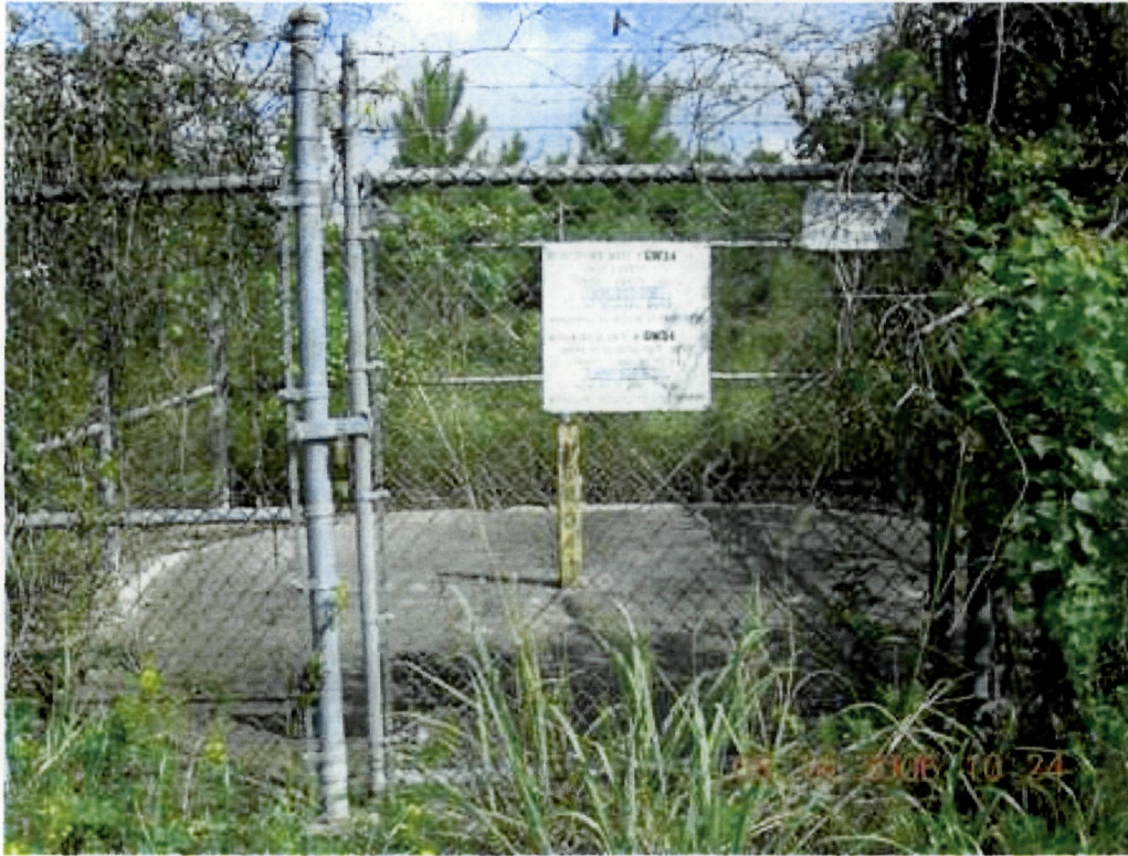
Photo 1: View of chain link fence at monitor well GW-34 facing northwest. Warning sign is still posted and in good condition.
