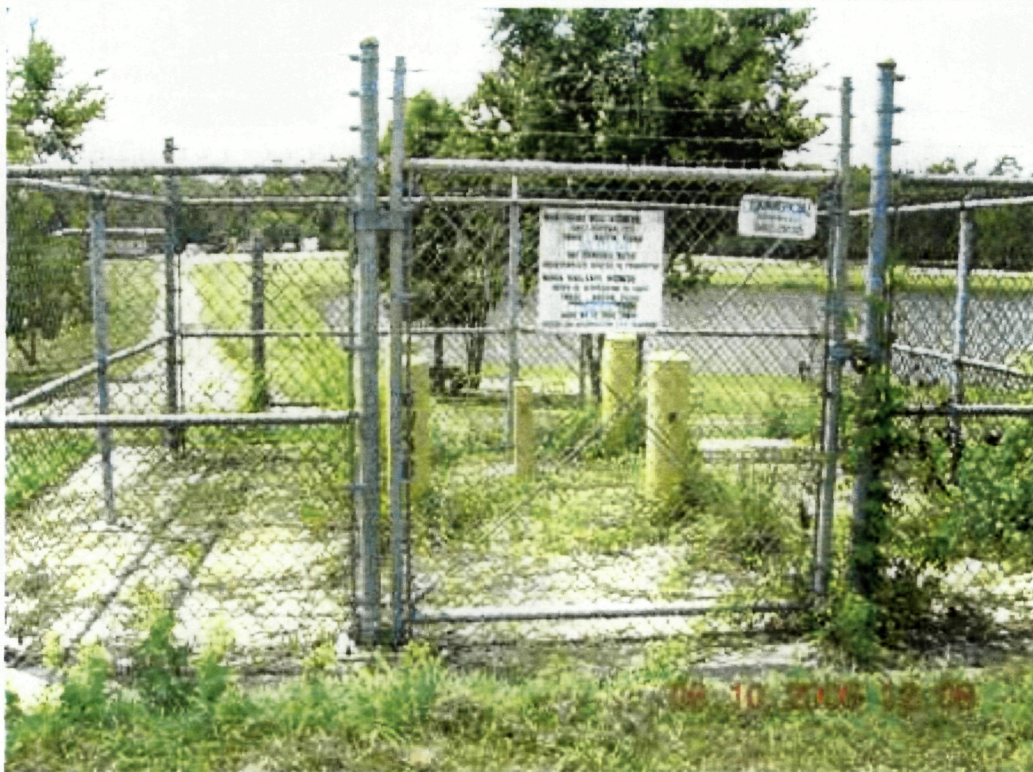
Photo 46: View of chain link fence at monitor well GW-30. Warning signs are posted and in good condition.
