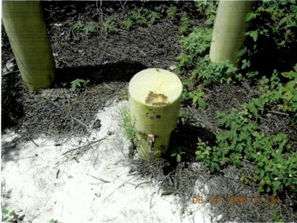
Photo 31: Protective casing at monitor well GW-21. The outer casing is properly secured.
