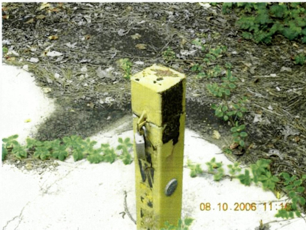
Photo 20: View of monitor well GW-35. The lock on the outer protective casing is broken at GW-35.
