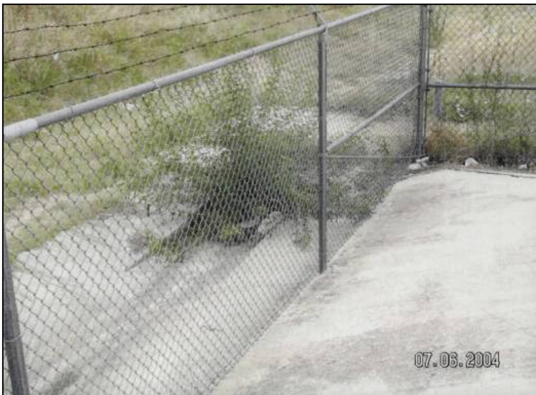
Small tree growing in a drain box Southeast corner of the Containment Cell
