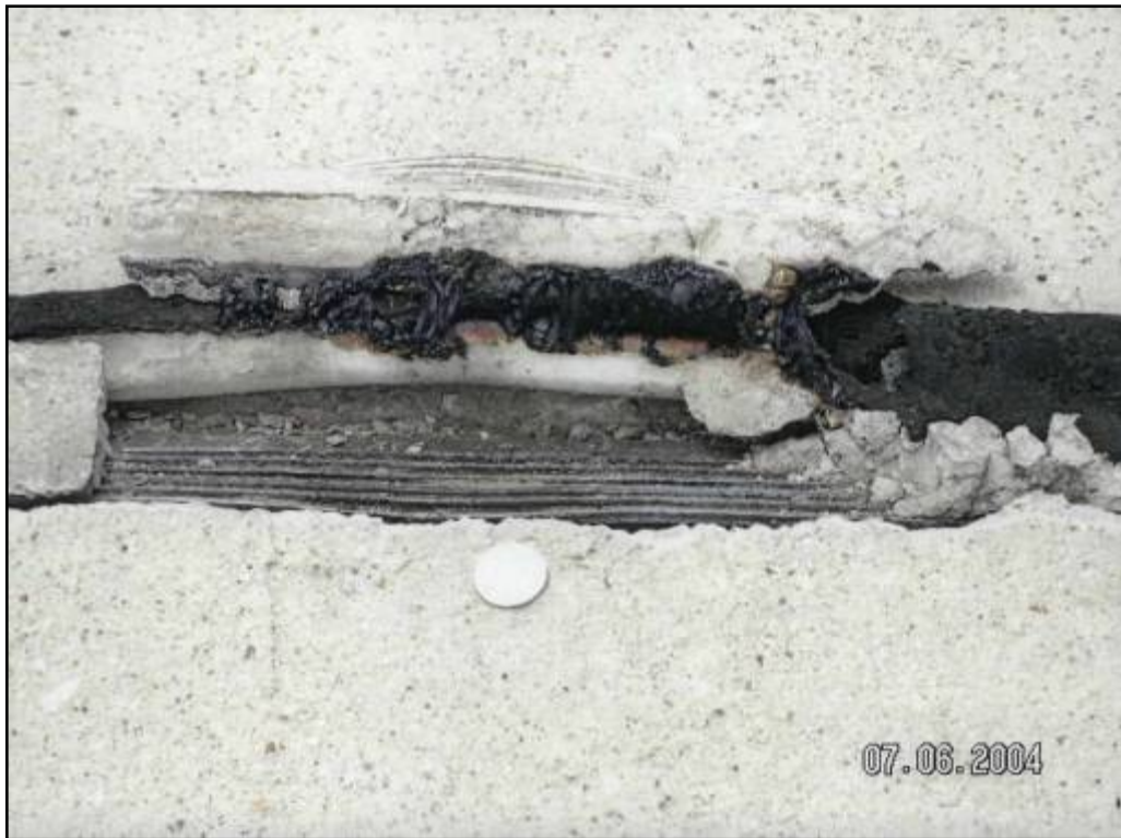
Containment Cell Cracked concrete at Crest Seam Foam Expansion joint visible
