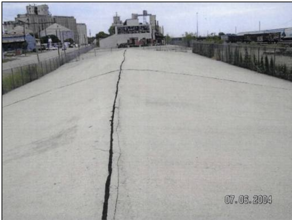
Containment Cell Cap Concrete Crack adjacent to Crest seam View to the North
