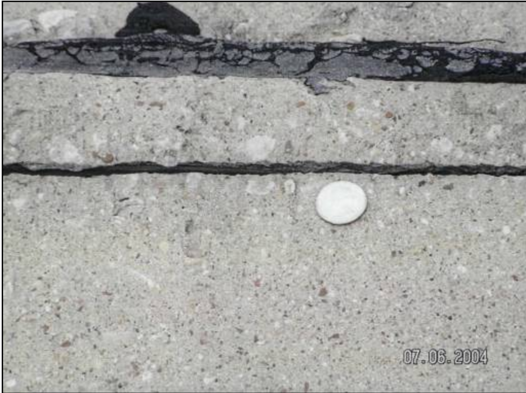
Containment Cell Concrete crack adjacent to Crest Seam
