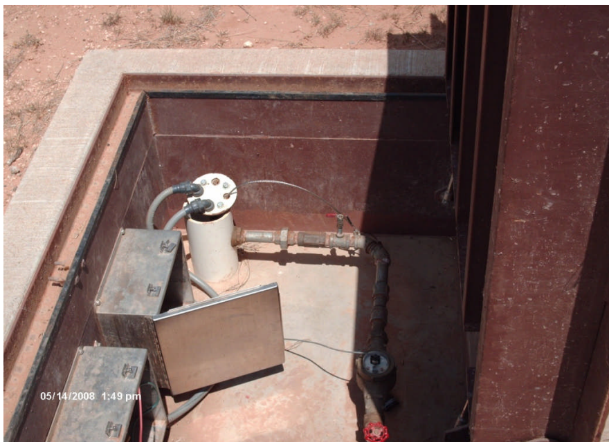
Photograph No. 8 Site: Sprague Road Ground Water Plume Superfund Site Description: View of wiring in extraction well NRW-13. The Coyote controller eliminates the need for relays in the vaults. Date: 14 May 2008
