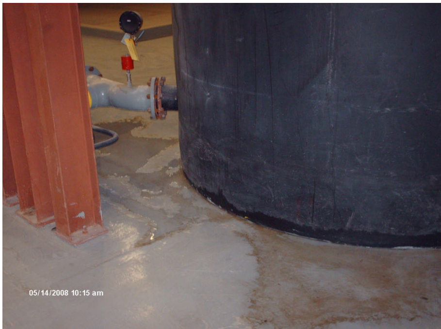
Photograph No. 2 Site: Sprague Road Ground Water Plume Superfund Site Description: Additional view of leaking Tank T-1A. Date: 14 May 2008
