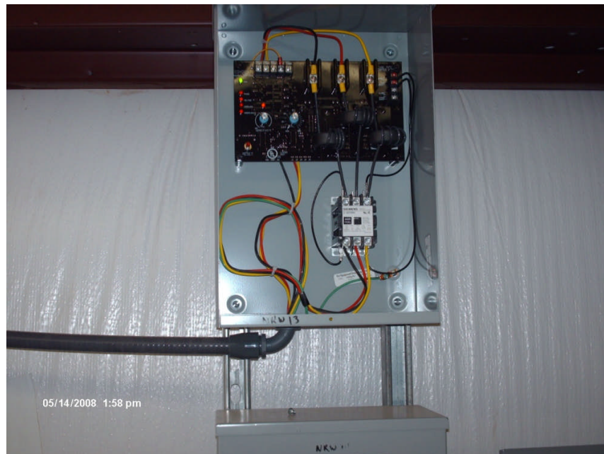
Photograph No. 9 Site: Sprague Road Ground Water Plume Superfund Site Description: View of Coyote control box for NRW-13 inside the NCC control building. Date: 14 May 2008
