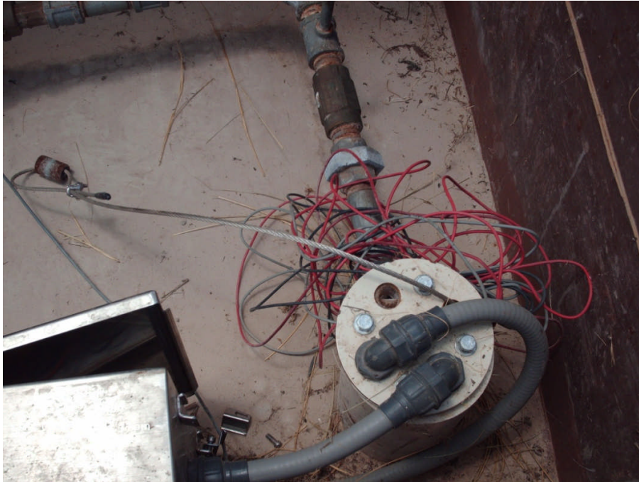
Photograph No. 5 Site: Sprague Road Ground Water Plume Superfund Site Description: View of wiring in extraction well MRW-2. Date: 14 May 2008
