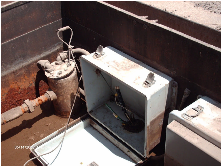
Photograph No. 7 Site: Sprague Road Ground Water Plume Superfund Site Description: View of wiring in extraction well NRW-17. The Coyote controller eliminates the need for relays in the vaults. Date: 14 May 2008
