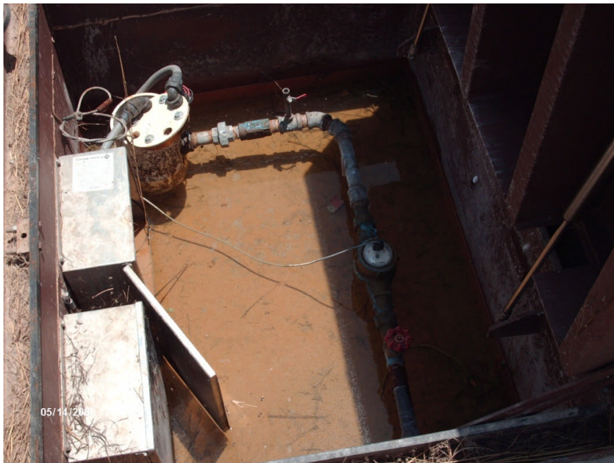
Photograph No. 6 Site: Sprague Road Ground Water Plume Superfund Site Description: View of flooded well vault in extraction well MRW-1. Date: 14 May 2008
