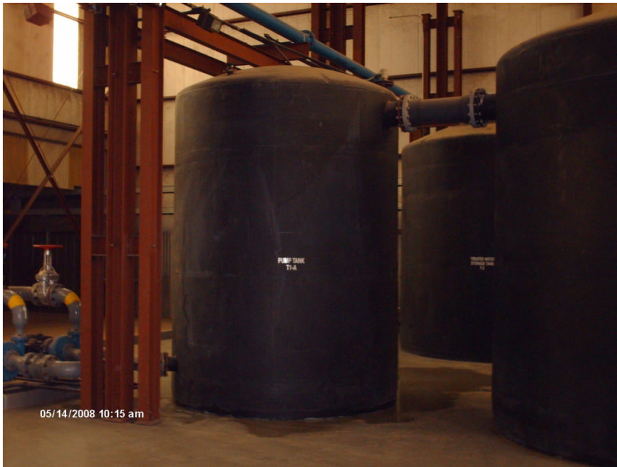
Photograph No. 1 Site: Sprague Road Ground Water Plume Superfund Site Description: View of leaking Tank T-1A inside the LM treatment facility. Date: 14 May 2008
