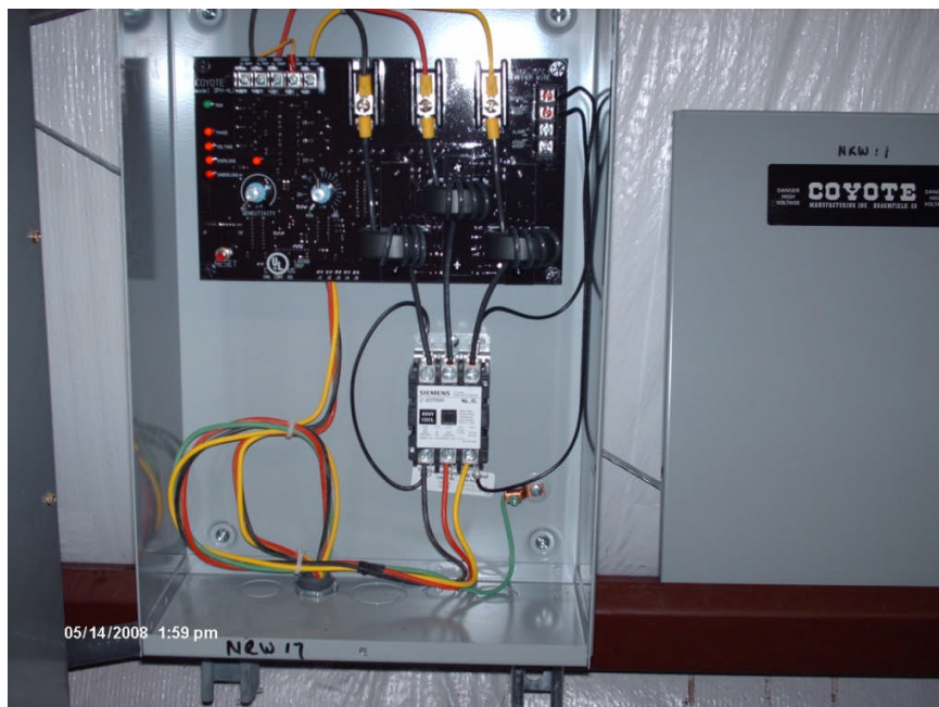
Photograph No. 10 Site: Sprague Road Ground Water Plume Superfund Site Description: View of Coyote control box for NRW-17 inside the NCC control building. Date: 14 May 2008
