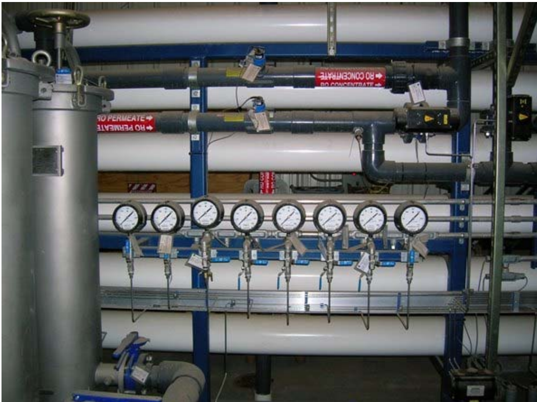
Photo 6: RO unit inside RO Facility.
