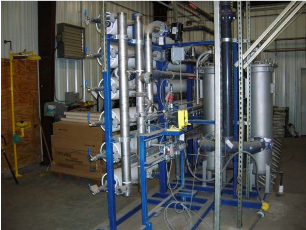
Photo 7: RO unit inside RO Facility.
