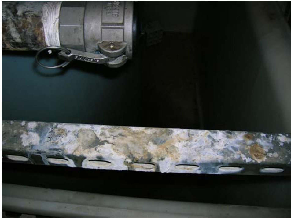
Photo 15: Acid staining from spills on the metal railing on secondary containment of the acid tank in ASTP.
