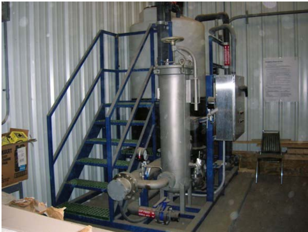
Photo 8: View of equipment inside RO Facility.
