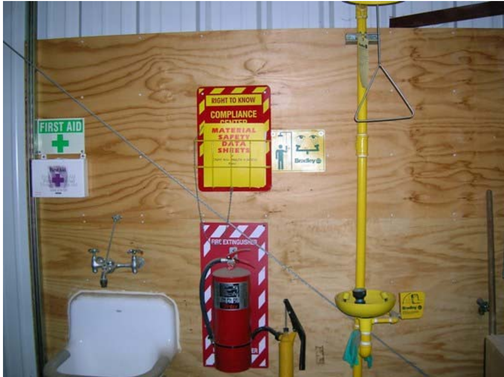
Photo 9: Safety equipment on wall inside RO Facility.
