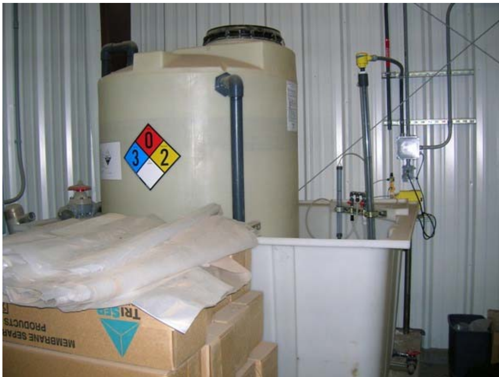
Photo 10: Caustic Soda tank inside RO Facility.
