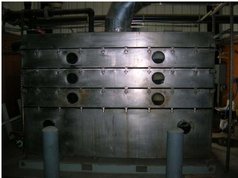
Photo 12: Air Stripper unit inside ASTP.
