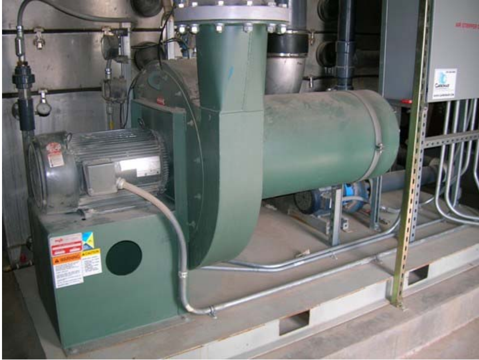
Photo 17: Blower unit in the ASTP.
