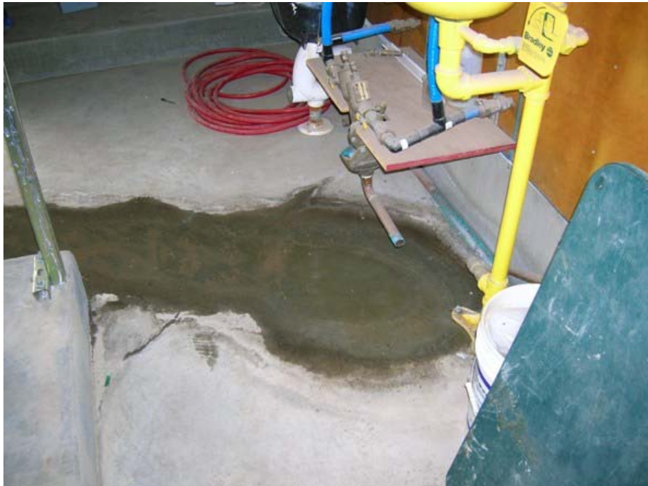
Photo 16: Leak on safety shower in the ASTP.
