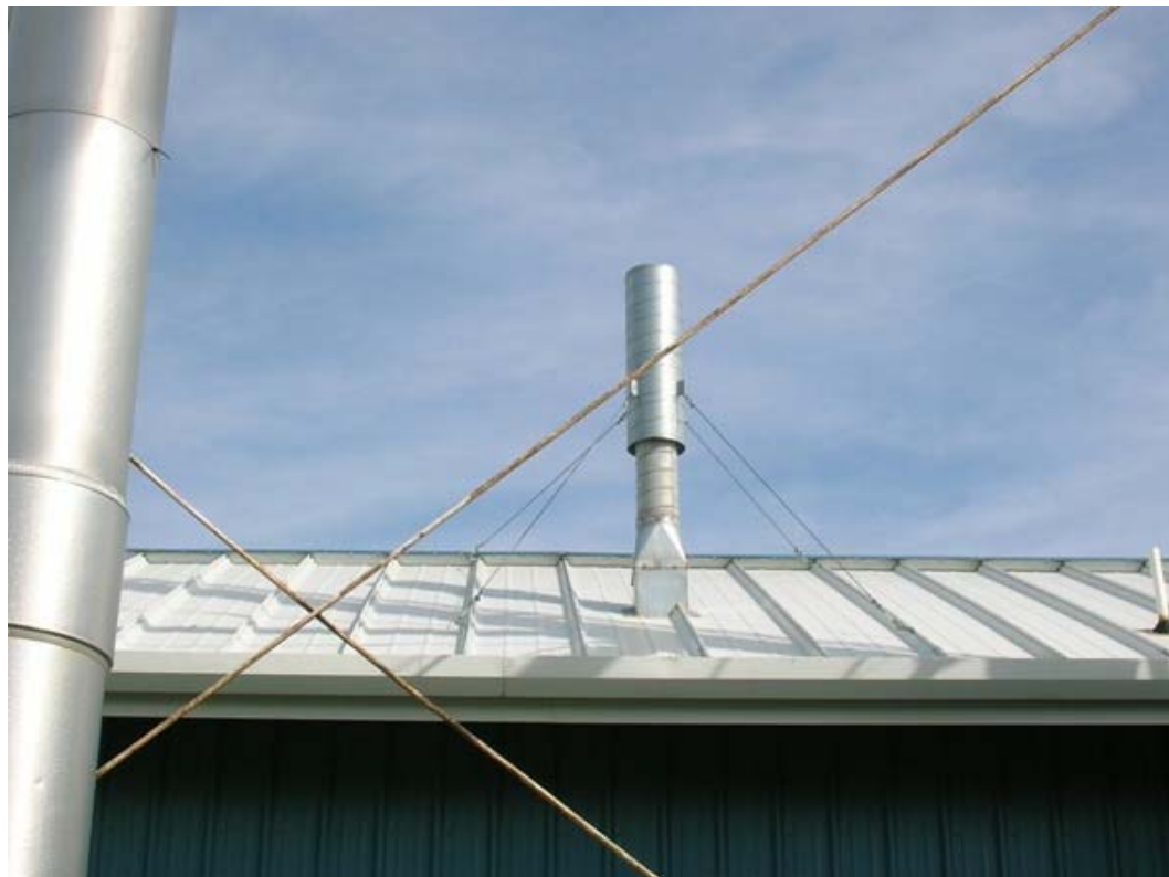
Photo 2: Air Stripper exhaust stack on top of ASTP building.
