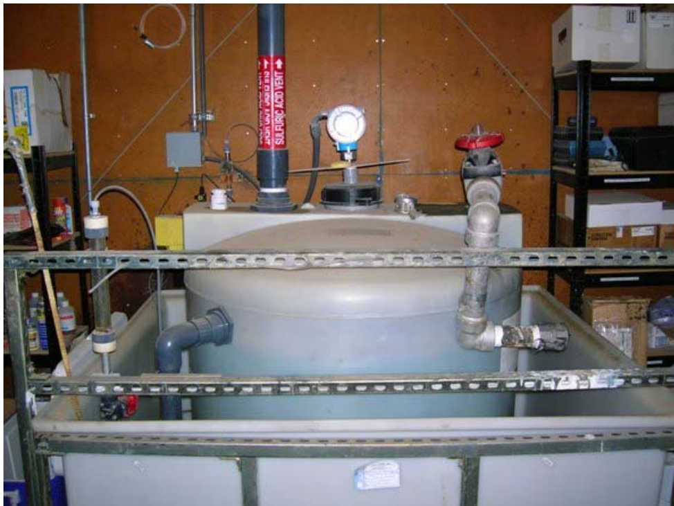
Photo 14: Sulfuric acid storage tank inside ASTP.
