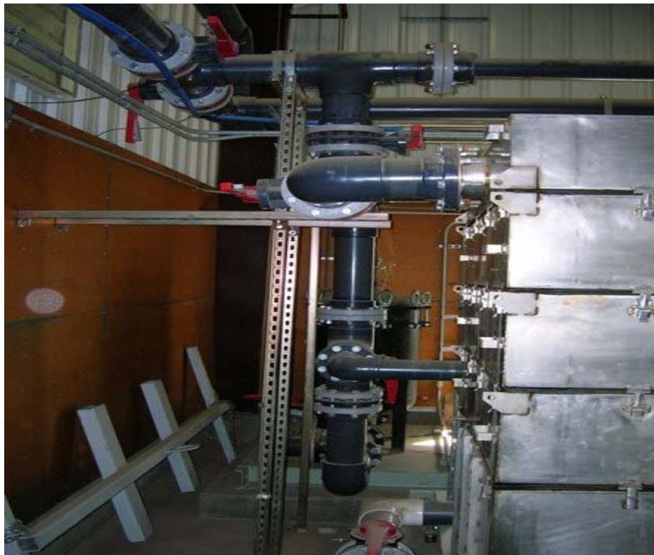
Photo 20: Piping on north side of air stripper in ASTP.
