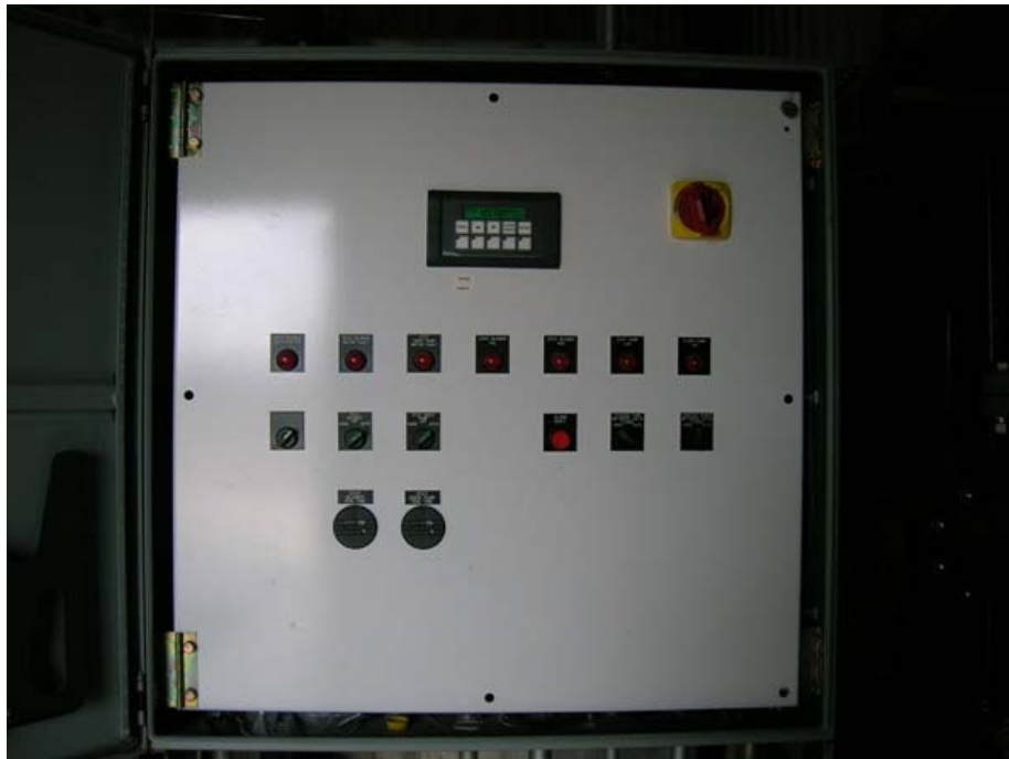
Photo 18: Instrument and Control panel in the ASTP.
