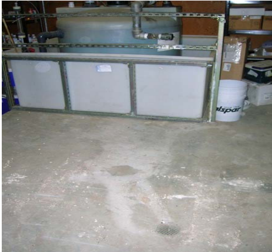
Photo 21: Acid staining on floor around acid tank in ASTP.
