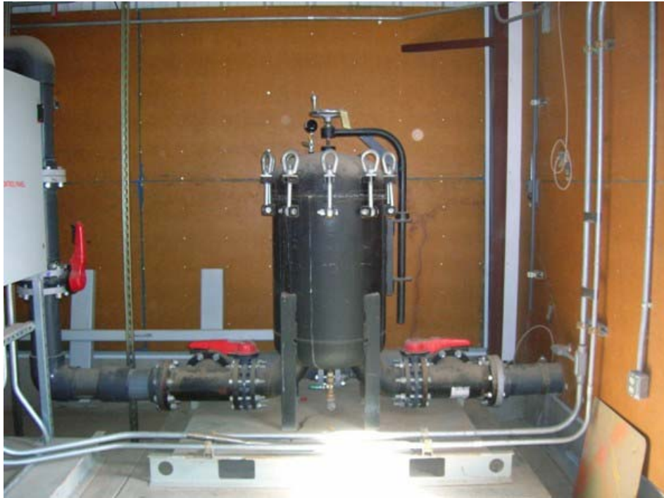
Photo 19: Bag filter in the ASTP. Water from the extraction wells enters from the right.
