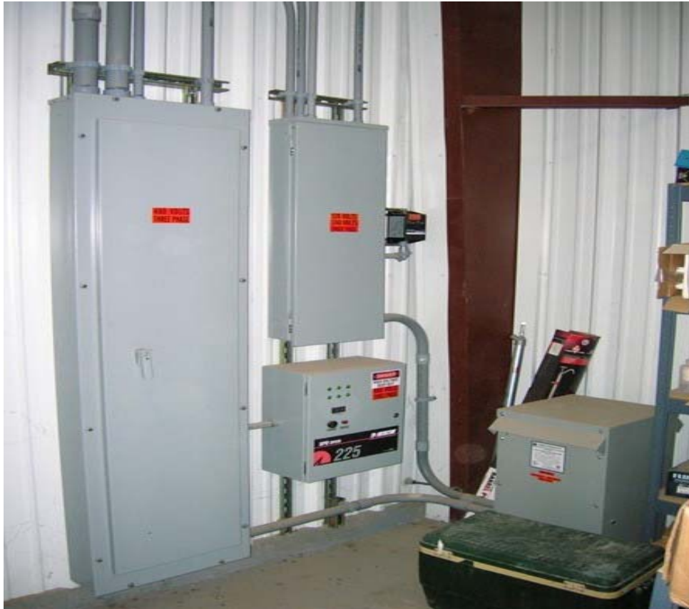
Photo 11: Instrument and Control panel in RO Facility.
