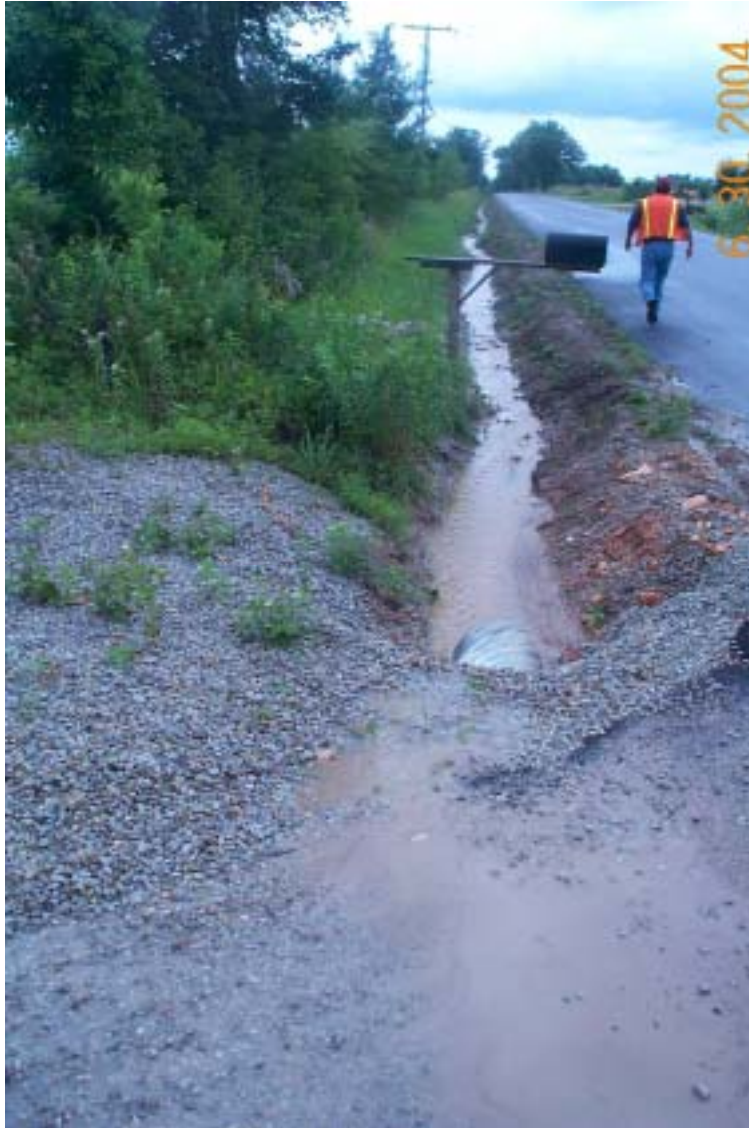
Photo 47: View upstream in the drainage ditch and culvert at entrance to borrow source. Runoff water in the drainage ditch is discolored from silt.
