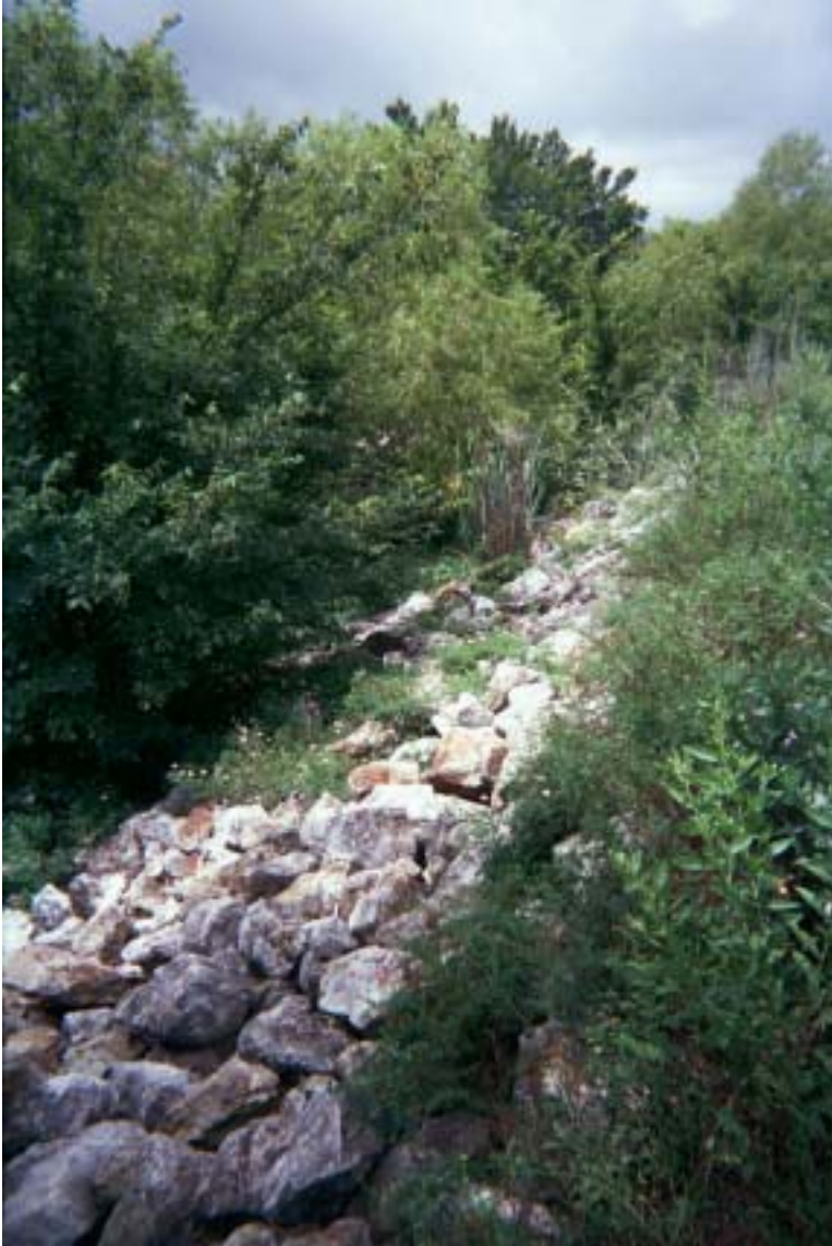
Photo 65: View of diversion dike at the Big John Mine site, located in Kansas. The subsidence feature is located to the right of this view. Large rocks were put in place to protect against erosion.
