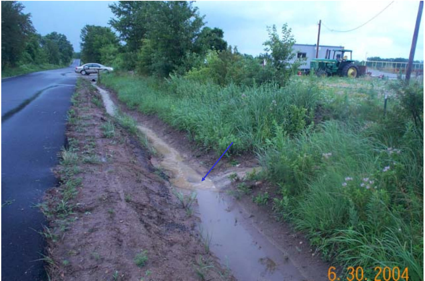
Photo 50: View of drainage ditch where runoff enters from the borrow source property. Discoloration of the runoff in the drainage ditch is apparent where the runoff enters the ditch (blue arrow).
