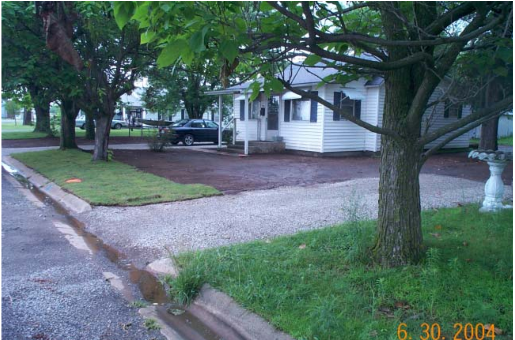
Photo 36: View of property in Commerce, Oklahoma. Construction was not complete at the time of the site inspection. Remediated portion of the yard (bare area in middle of photograph) is awaiting the placement of sod.
