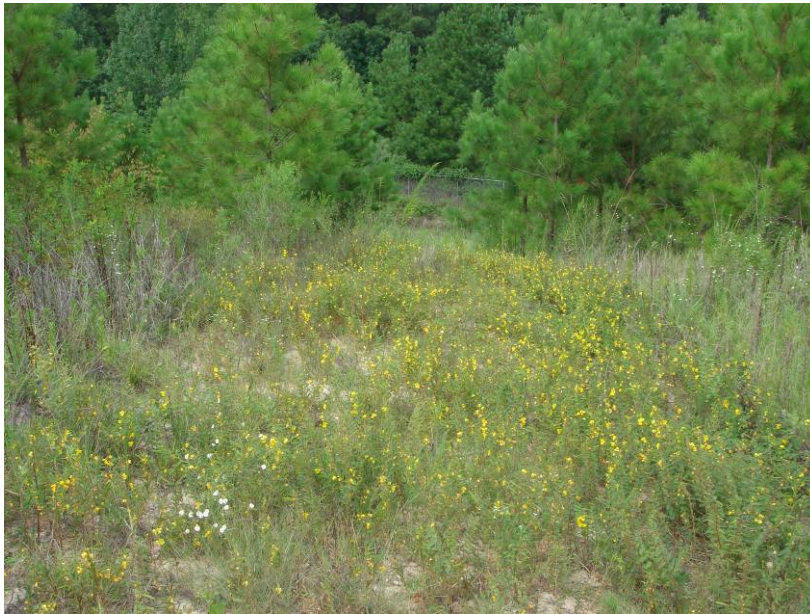
Photo 4. Eroded area on top of landfill cell. Picture taken facing east in September 2006.
