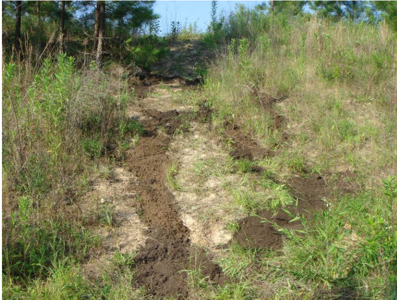
Photo 1. The eroded area was backfilled with dirt and re-seeded. Picture taken facing west in May 2006.
